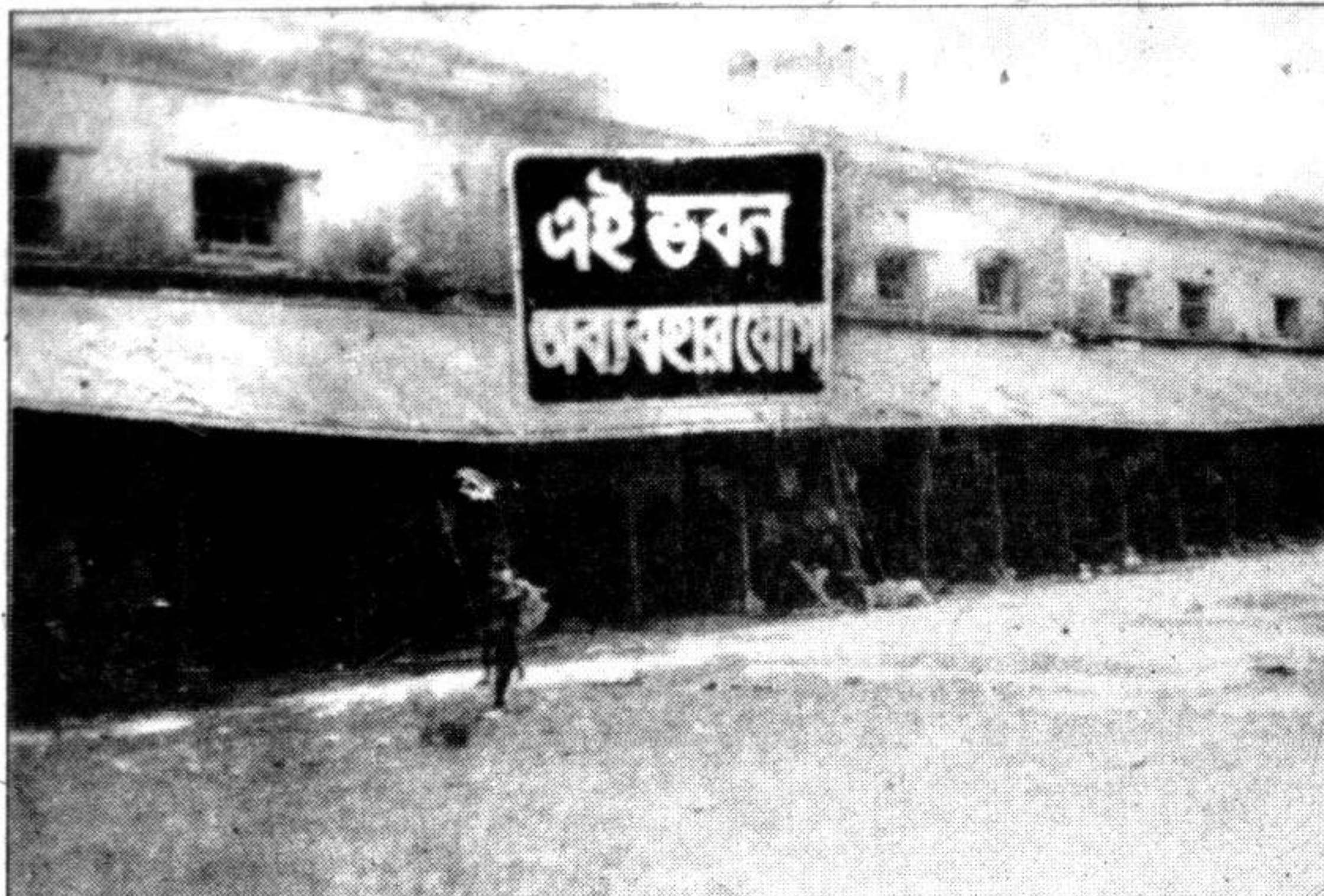
NATORE: Many rootless people are at present residing in the dilapidated and abandoned court building of the district risking their life. — Star photo
