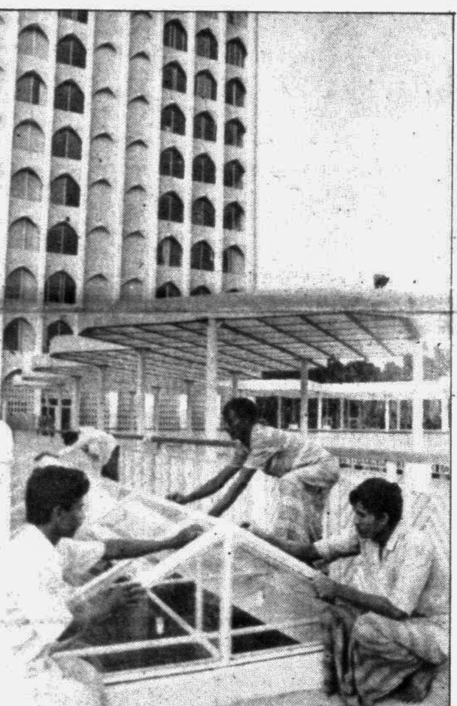
Dhaka Sheraton Hotel, the venue for the Seventh SAARC Summit is being given a face lift. — Star photo
