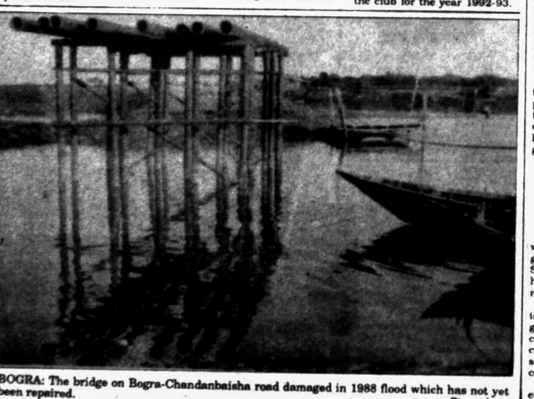
BOGRA: The bridge on Bogra-Chandanbaisha road damaged in 1988 flood which has not yet been repaired.
