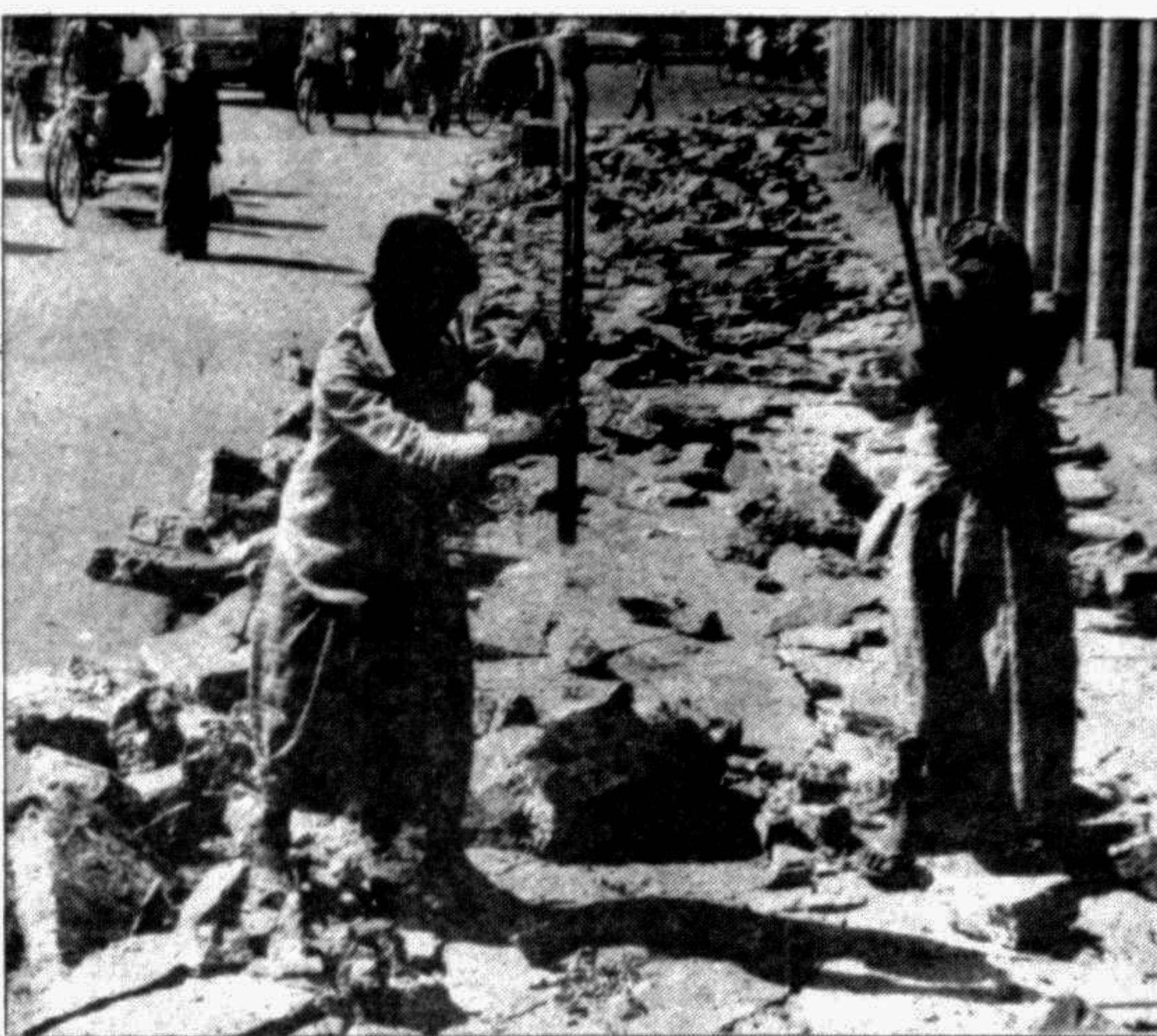
The foot-path adjoining the Ministry of Foreign Affairs building seemingly in 'good condition' being dismantled yesterday for 'repair'. — Star photo
