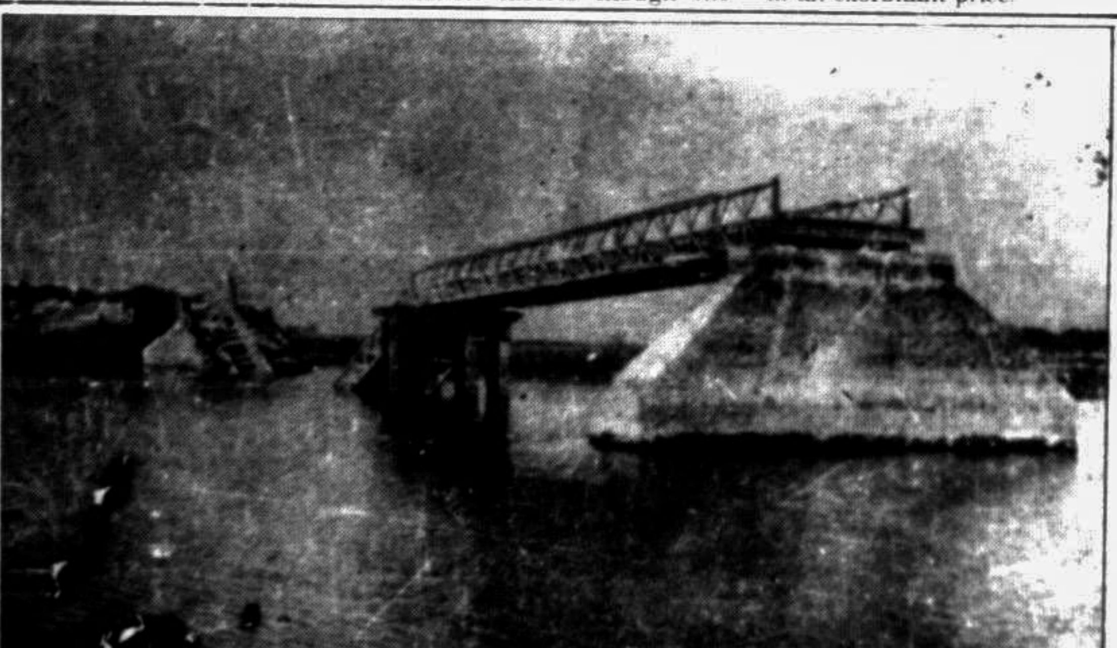
JAMALPUR: The baily bridge on Jamalpur-Madarganj Road damaged during 1988 flood has not yet been repaired. — Star photo
