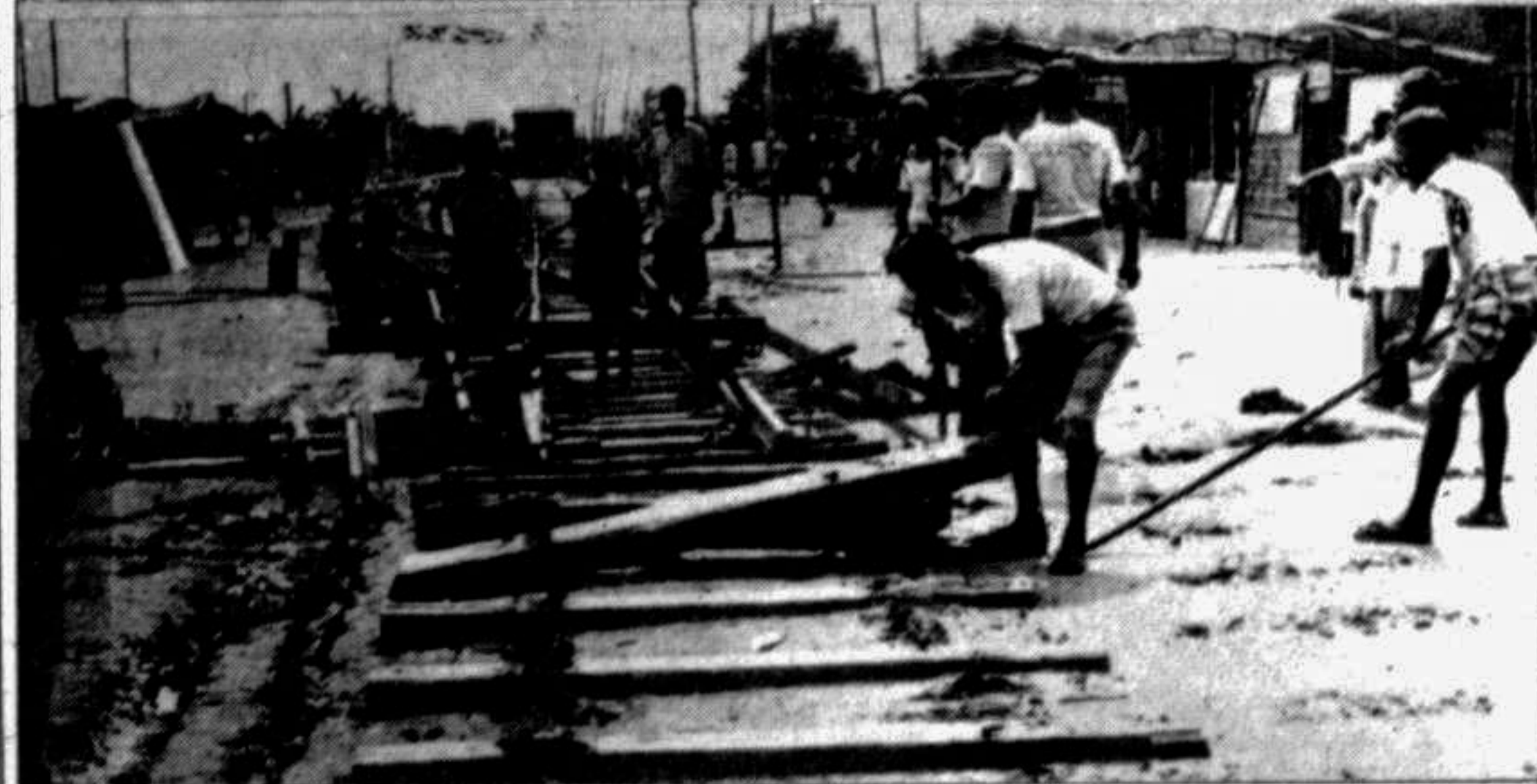
RANGPUR: The railline at Fulchari ghat in being repaired as it was damaged by a heavy shower recently. —Star photo
