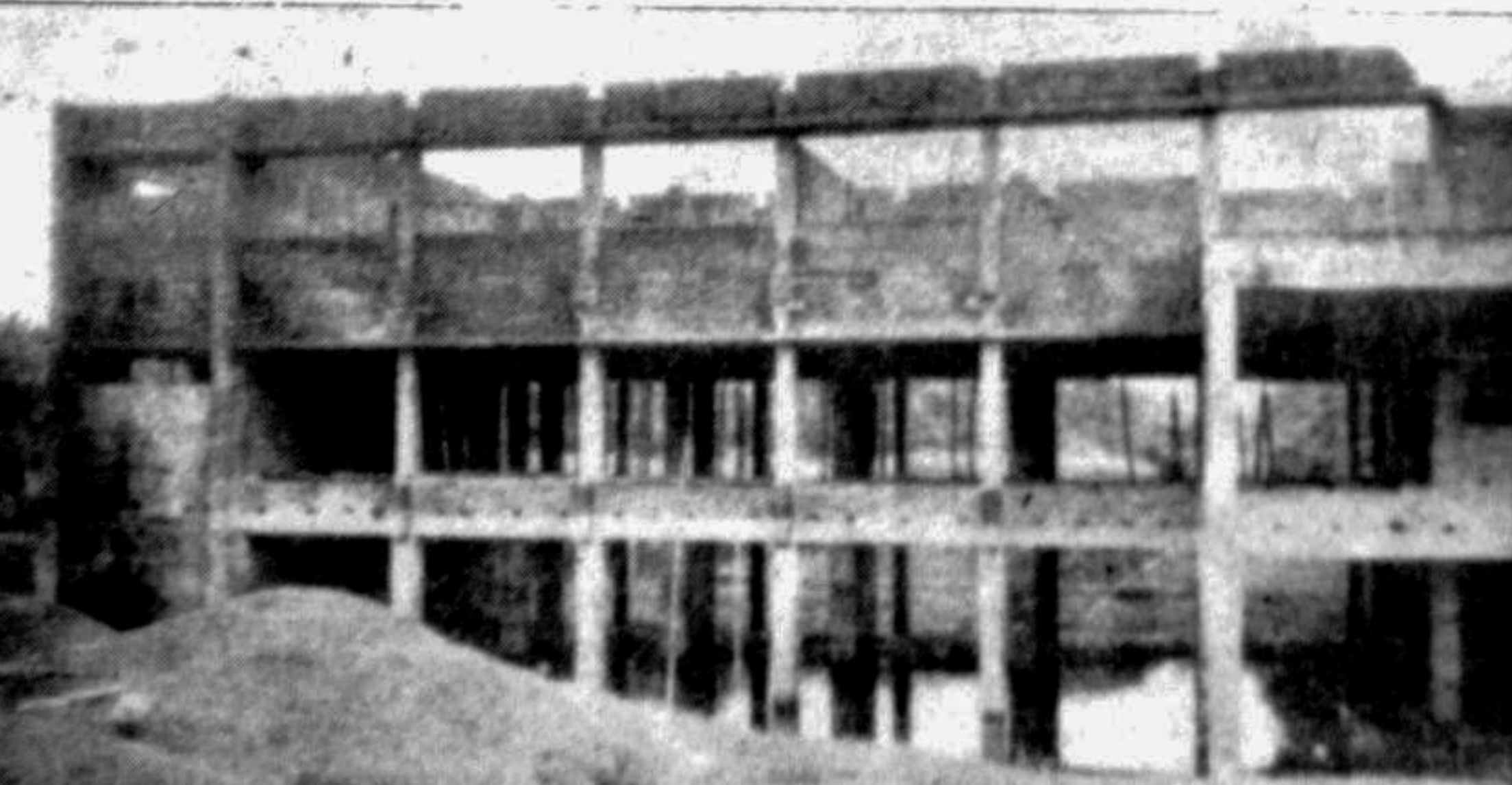
CHANDPUR: The office-building of the Superintendent of Police remains incomplete for years together. — Star photo
