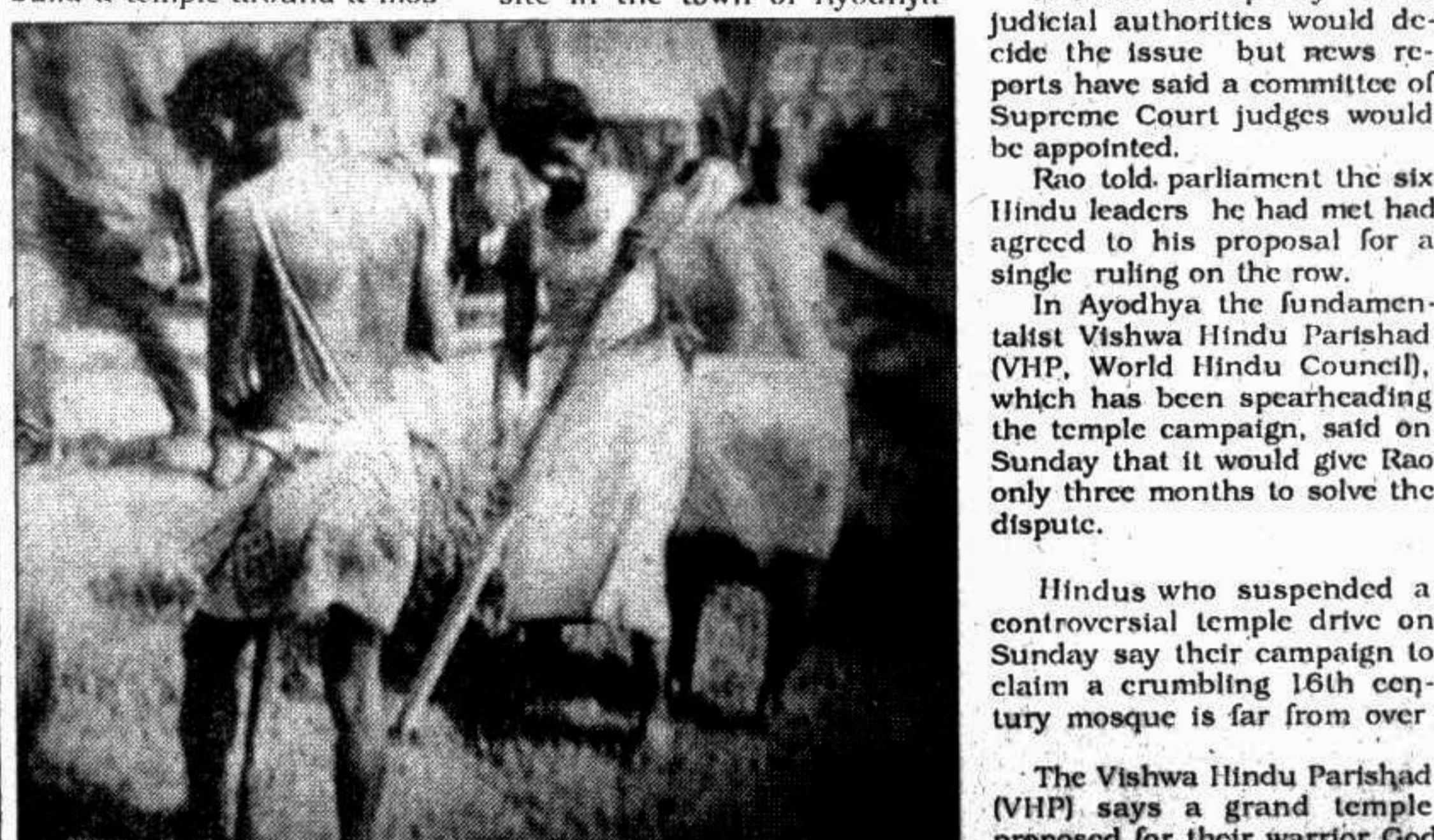
Militant Hindu activists working on a new site to construct a temple to be called 'Laksman Temple'. — TV photo
