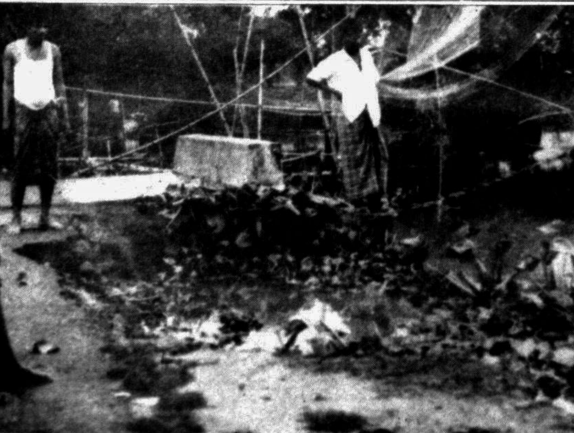
SYLHET: A culvert, newly constructed few days back on Chalibandar-Chhararpar Road of the town recently damaged for faulty construction. — Star photo
