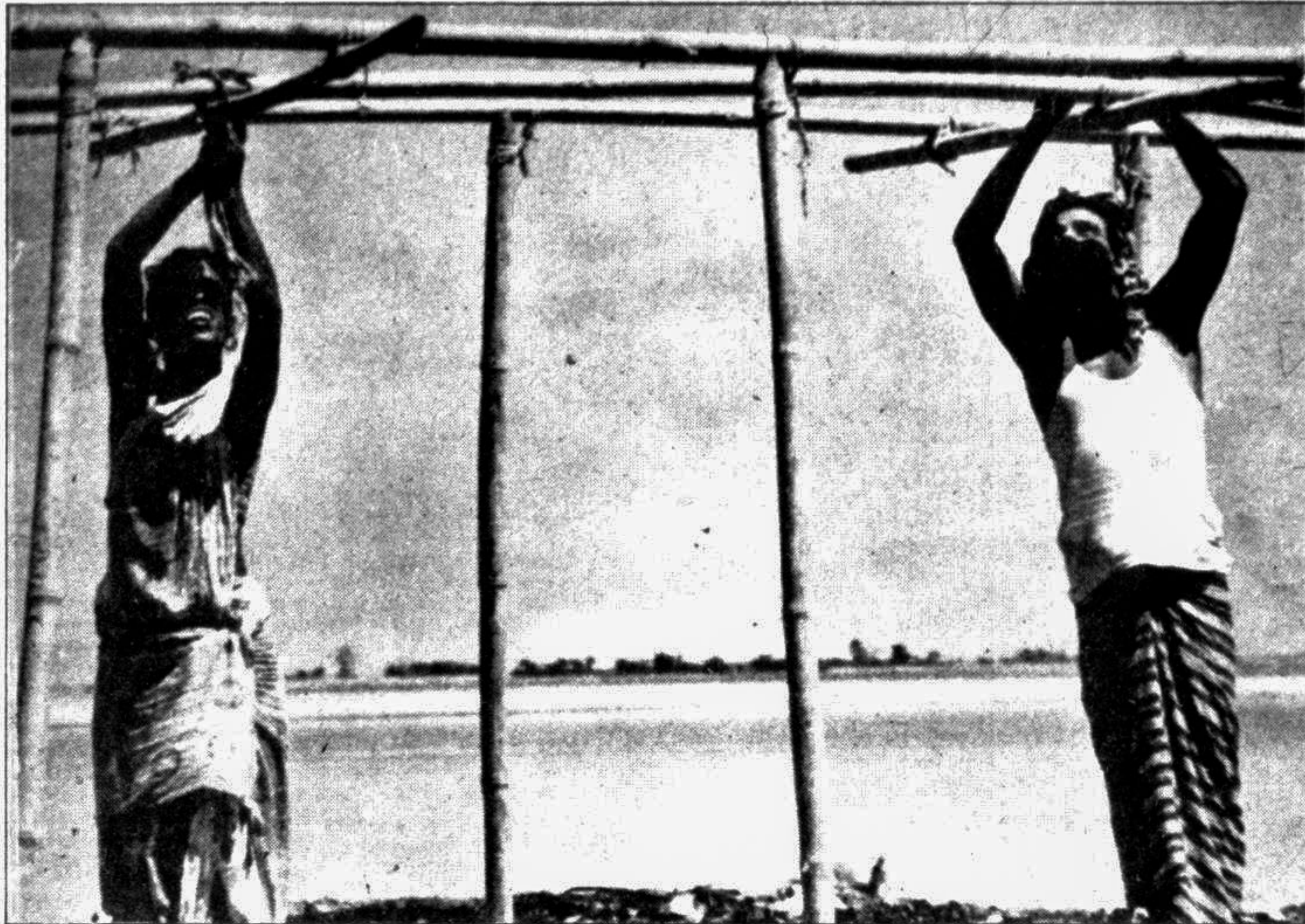
BOGRA: Husband and wife of a erosion-hit family of Shariakandi Upazila are making a shelter on the embankment to live in. — Star photo
