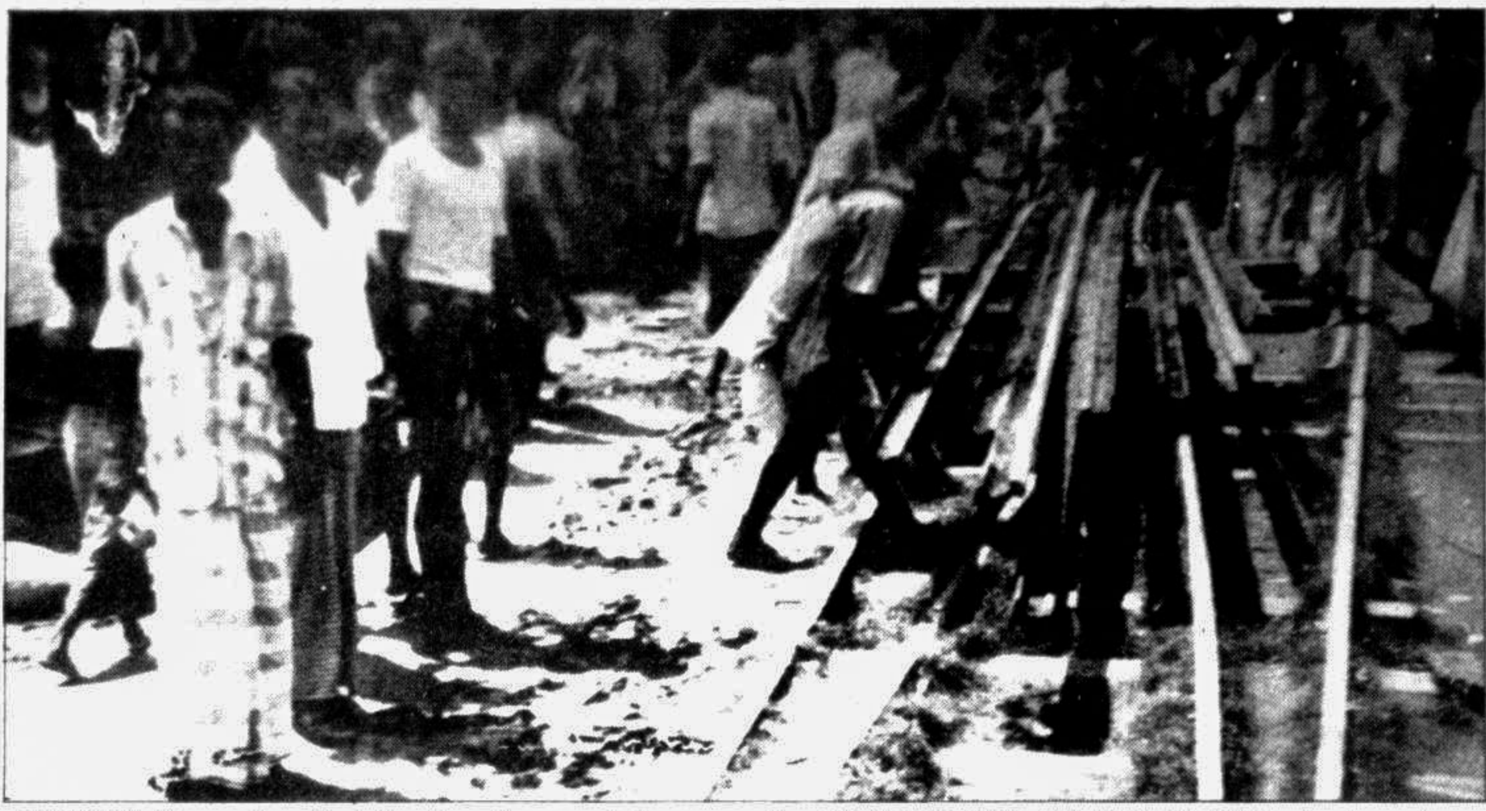
RAJBARI: The erosion affected railway lines are being removed on Bhatiapara route and the local station is also under threat. — Star photo
