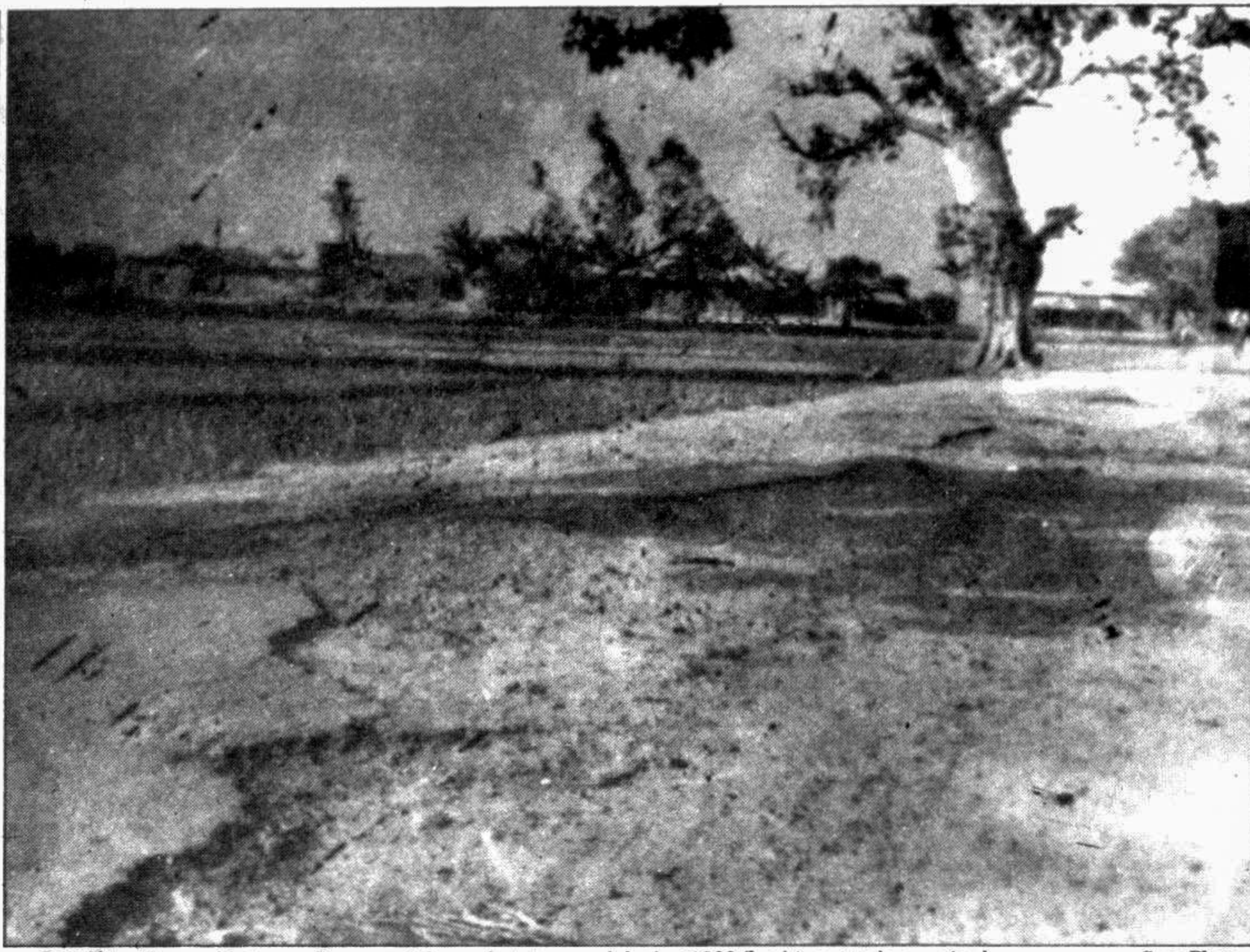
BOGRA: The road between Bogra and Joypurhat damaged during 1988 flood is yet to be repaired.
