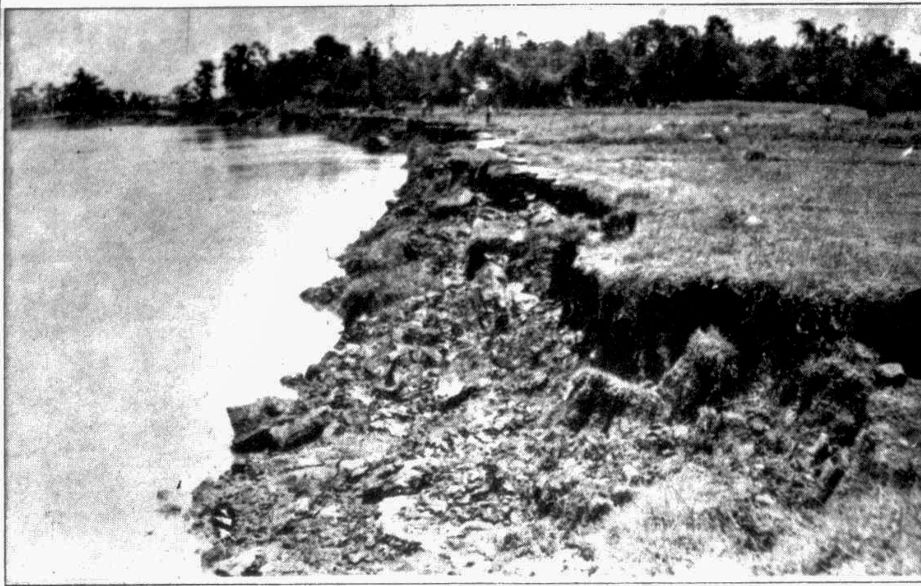
SYLHET: An erosion-hit village in Balaganj Upazila of the district.
