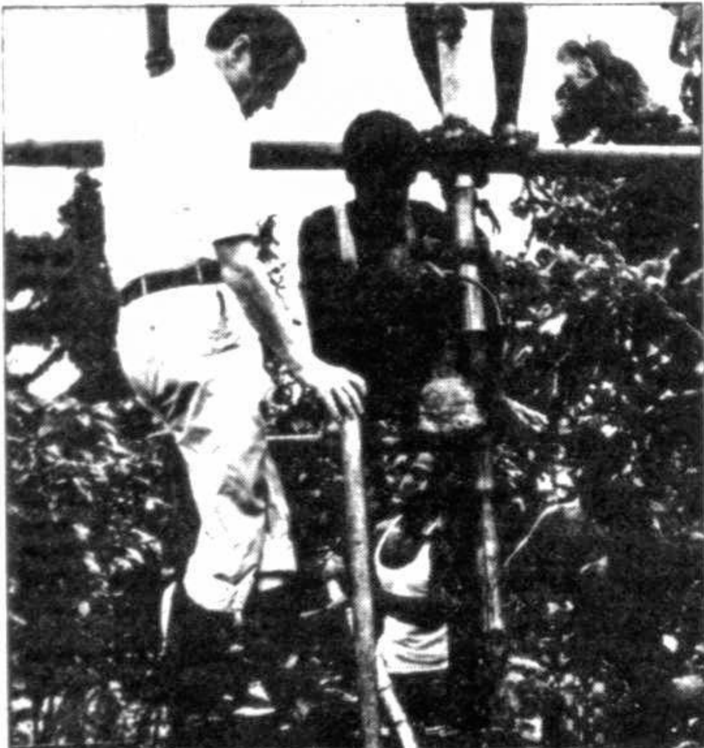
Mr James P Grant observes sinking of a tubewell under slinger method of tubewell construction at Savar near Dhaka in July 1980.
