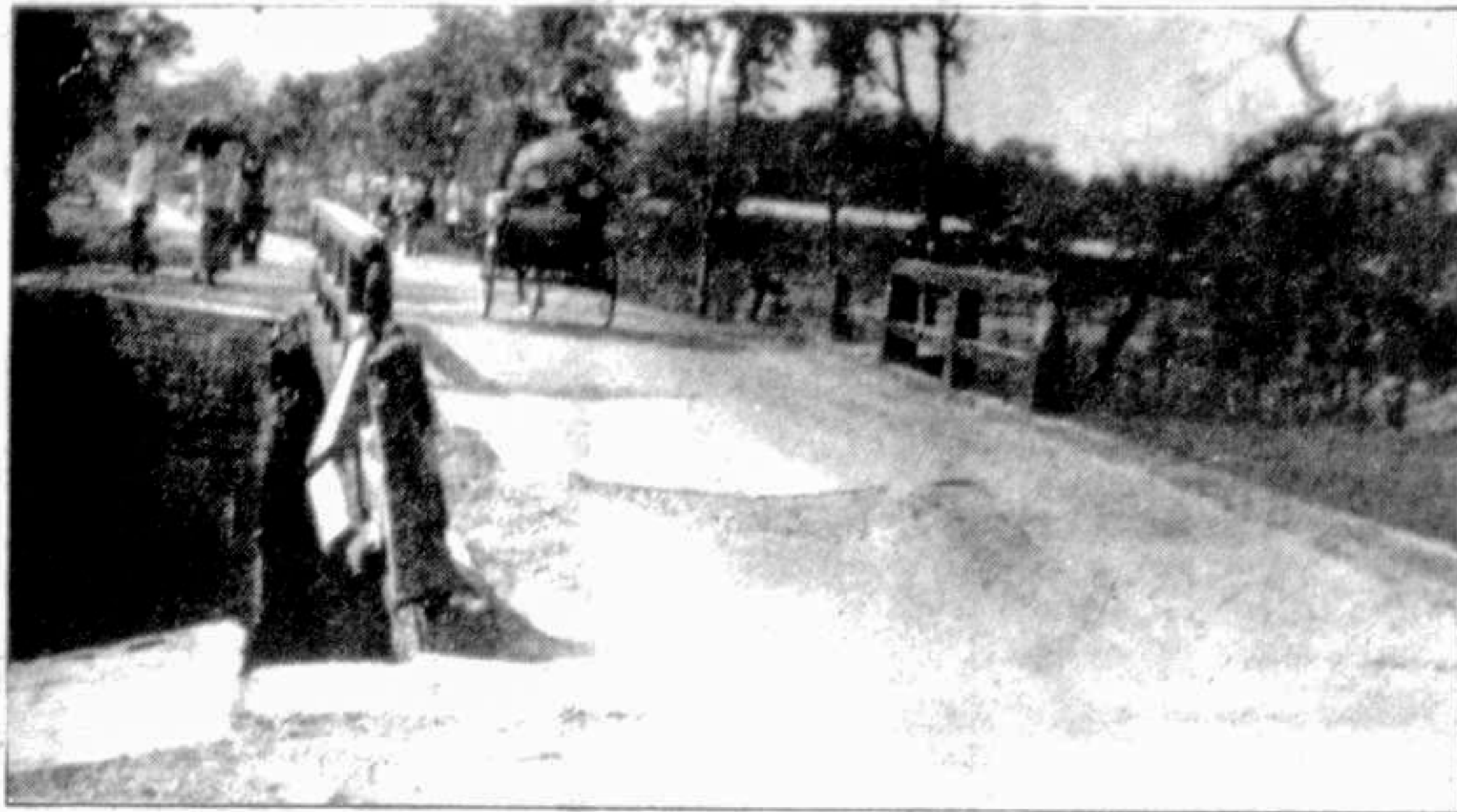
CHANDPUR: The bridge on Chandpur — Comilla Highway near Chandkhar Pool needs early repair to avoid mishap. — Star photo
