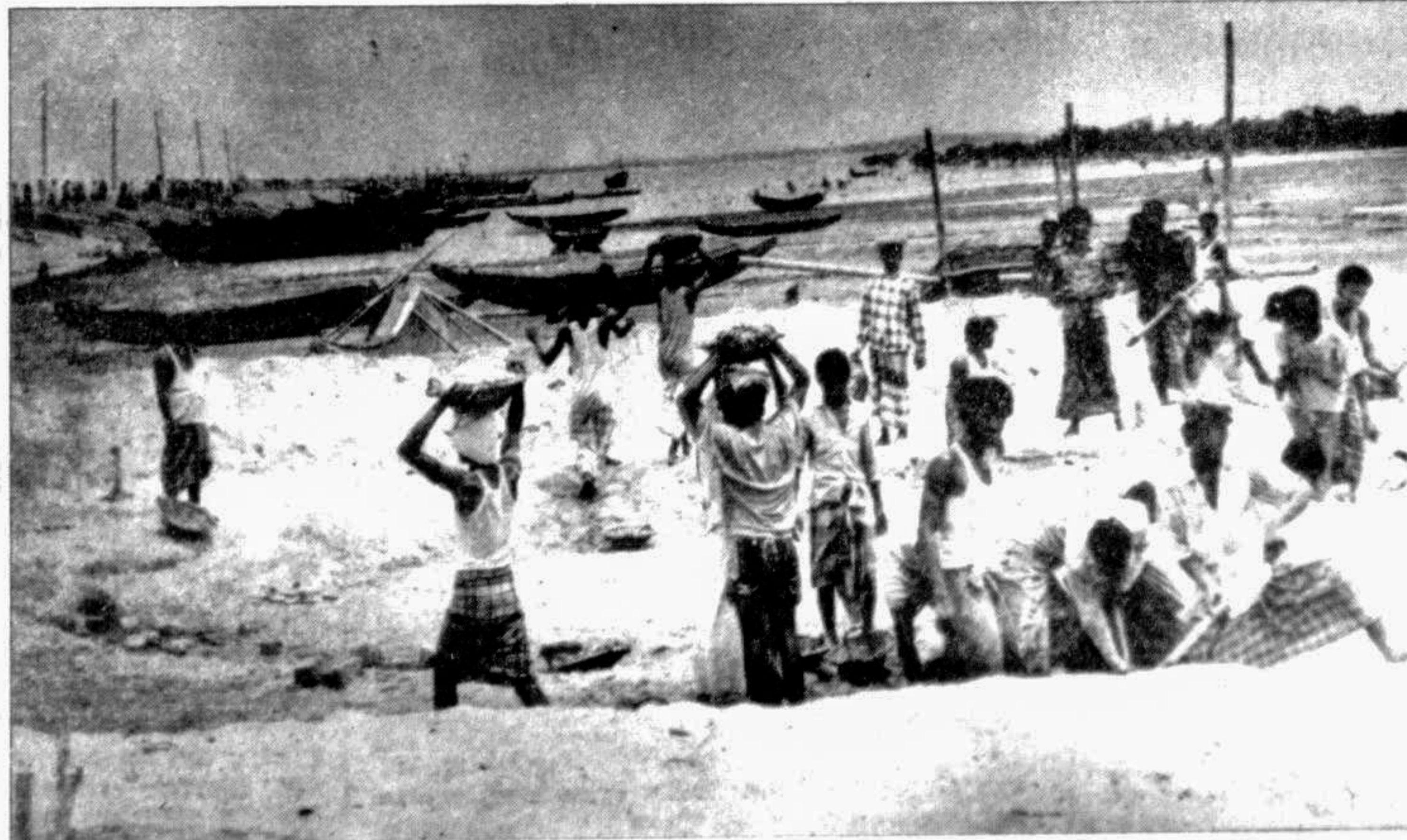
Right on the water's edge, a new cyclone shelter is being built at Ghorokkata Union of Maheshkhali. Although work was supposed to be completed by May this year, the contractors started work in the last week of April.
