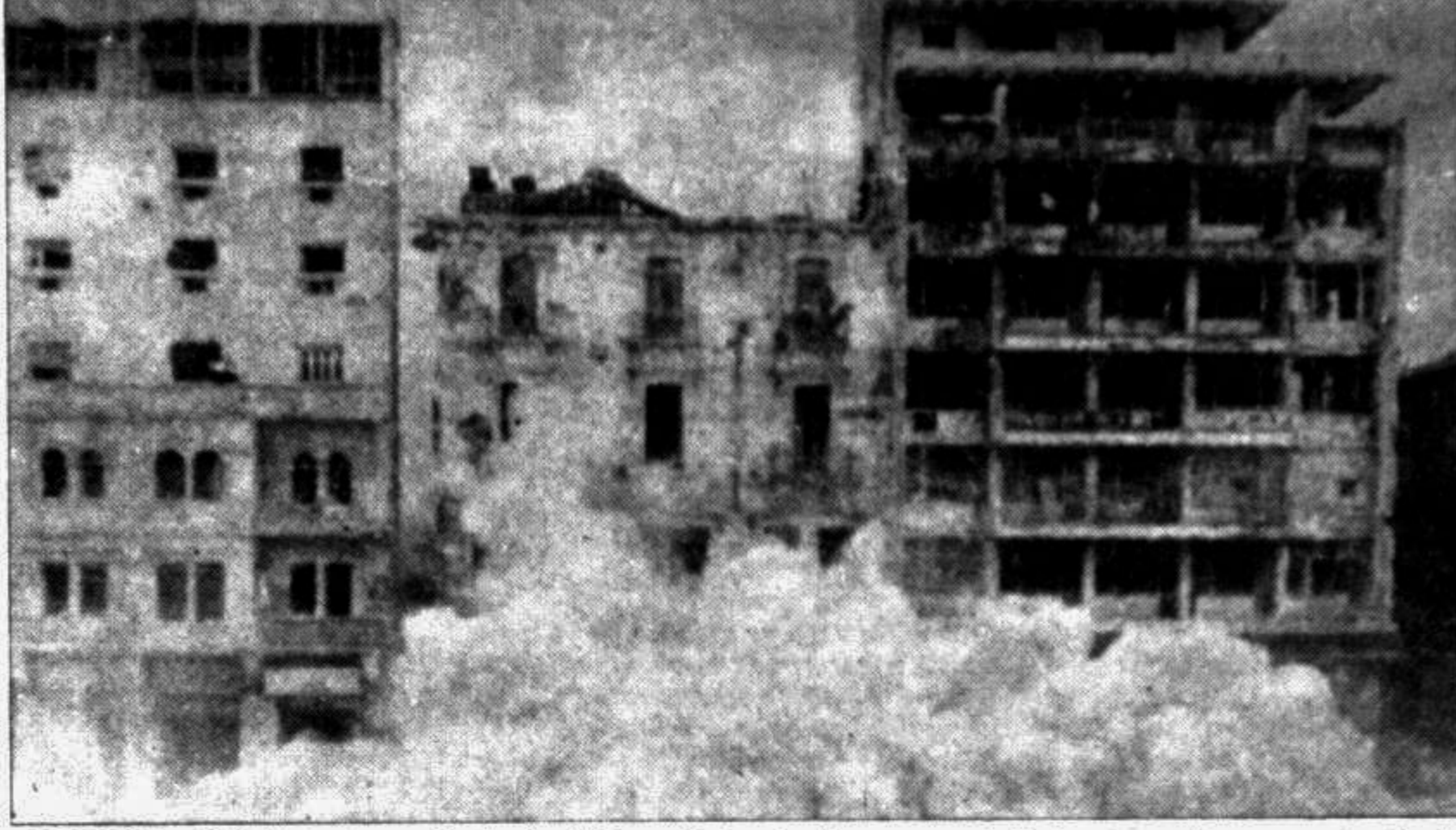
BEIRUT: Old Beirut market's building slides to the ground Saturday after a controlled explosion continued demolition work in the Lebanese capital.
