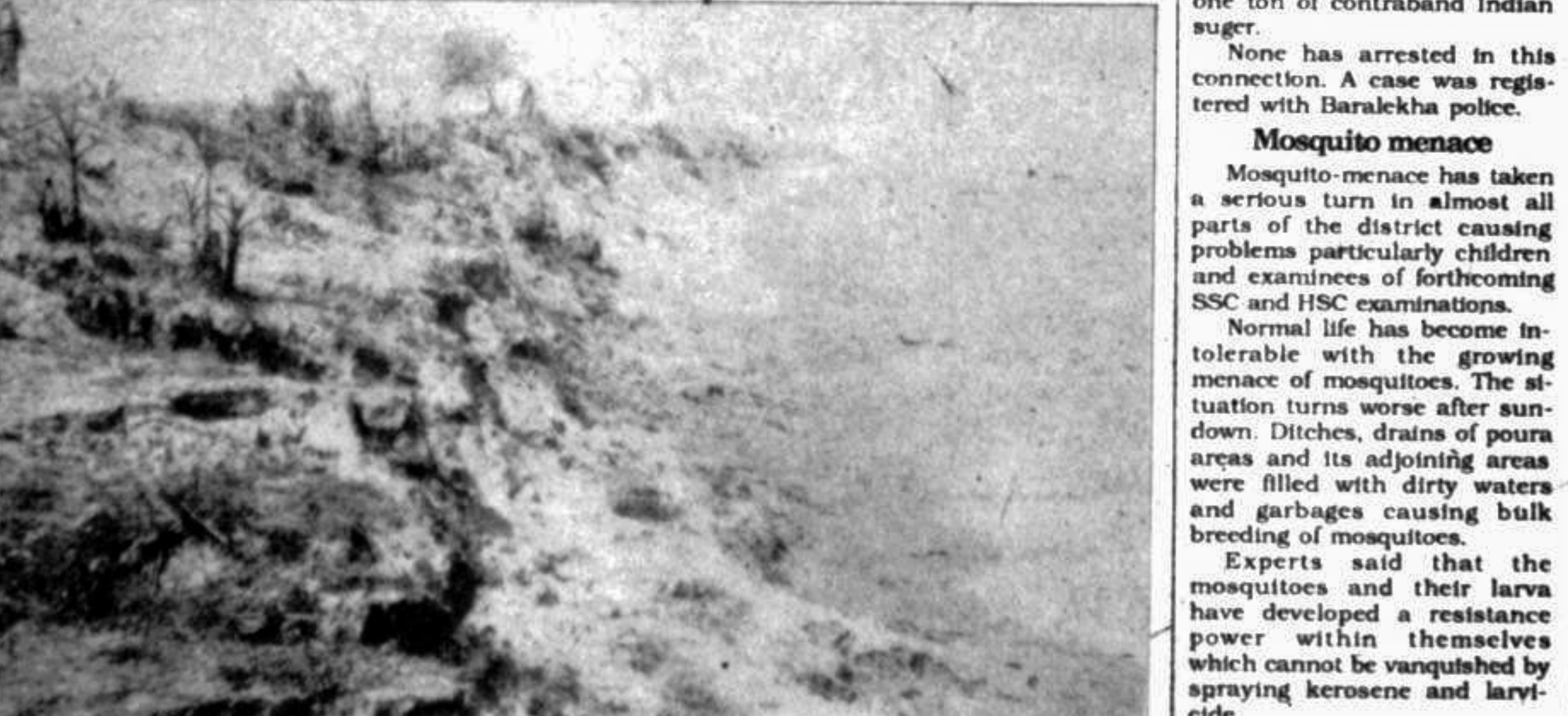
BOGRA: The embankment at Shariakandi to control flood and erosion of the river Jamuna is being damaged every year and thousands of people become landless. —Star photo
