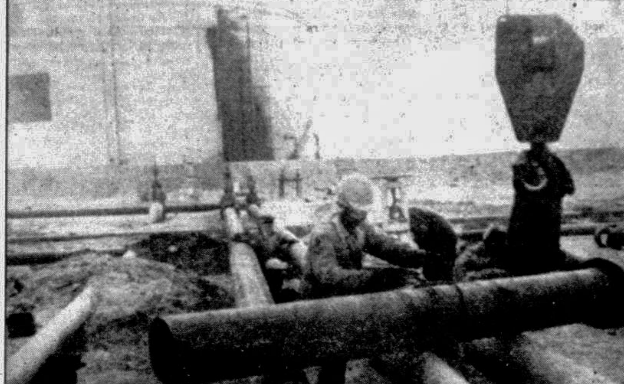
KUWAIT CITY: Workers fixing oil pipes at Wafra oil plant. Oil production from on-shore wells in the neutral zone between Saudi Arabia and Kuwait resumed Wednesday for the first time since the Gulf crisis. —AFP photo.
