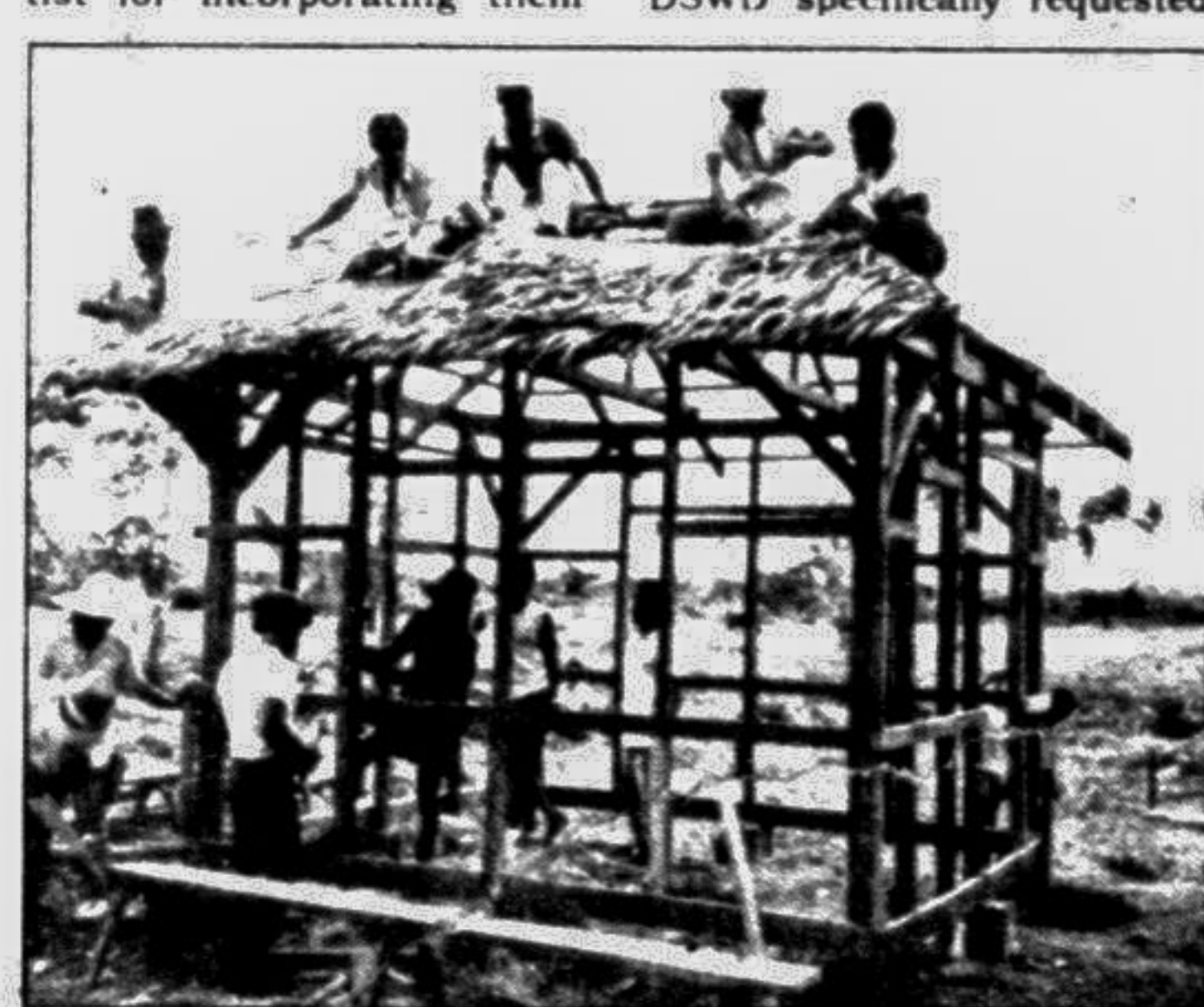
Locally available material "Nipa" being used by beneficiary for roof covering immediately after core construction.
