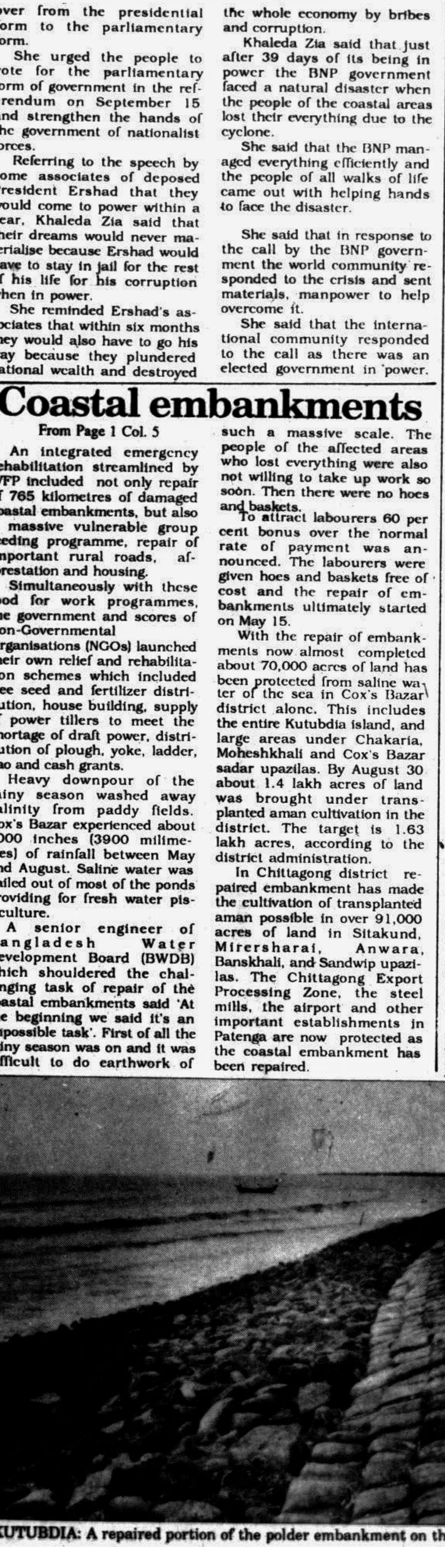
KUTUBDIA: A repaired portion of the polder embankment on the western side of Kutubdia. — Star photo by MK Majumder
