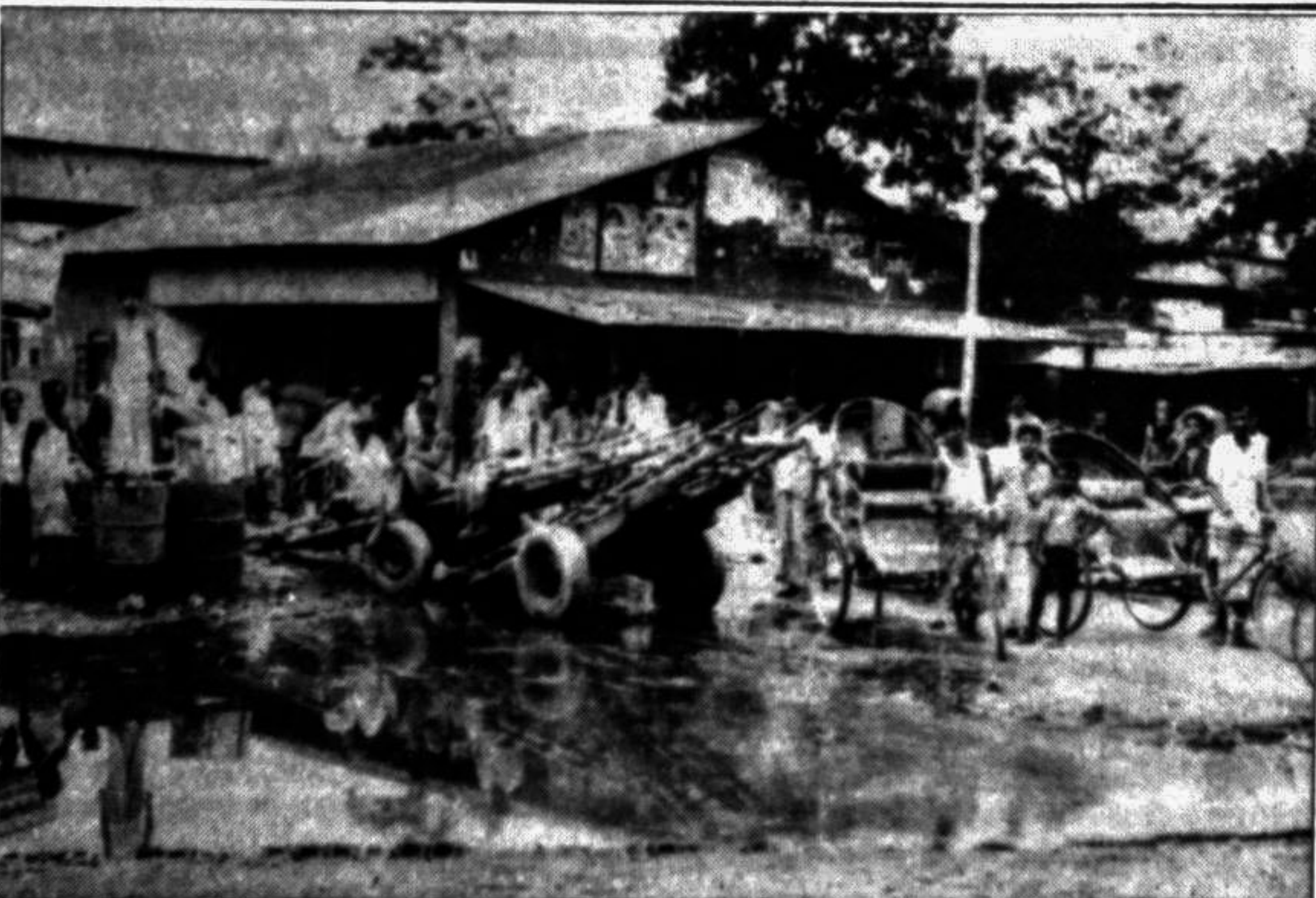
SIRAJGANJ: A big hole developed on Sirajganj Bazar railway station road posing threat to vehicular movement.
