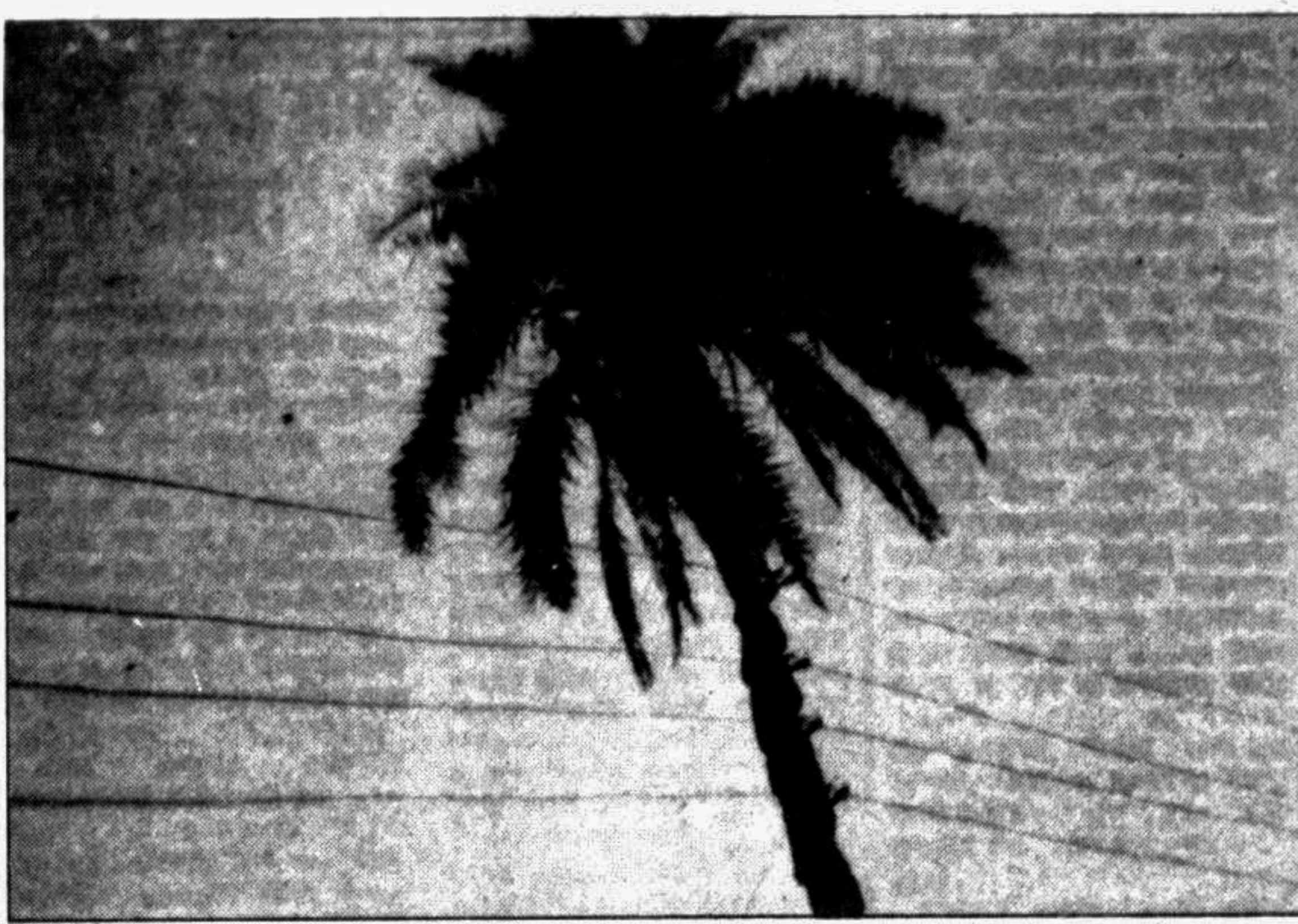
PABNA: Power Development Board has used many trees instead of poles to expand electric line at maligacha union under Pabna Sadar upazila posing danger to the villagers. —Star photo
