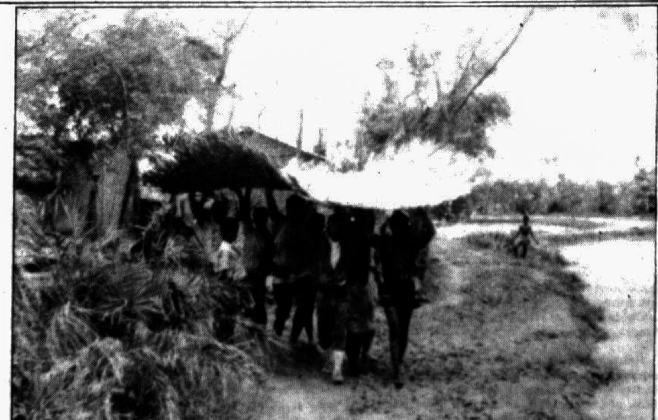
CHITTAGONG: Volunteers of Asian Friendship Society Bangladesh erecting houses at village Gahira (Hariarpara) under Anowara Upazila for the cyclone victims. — Star photo
