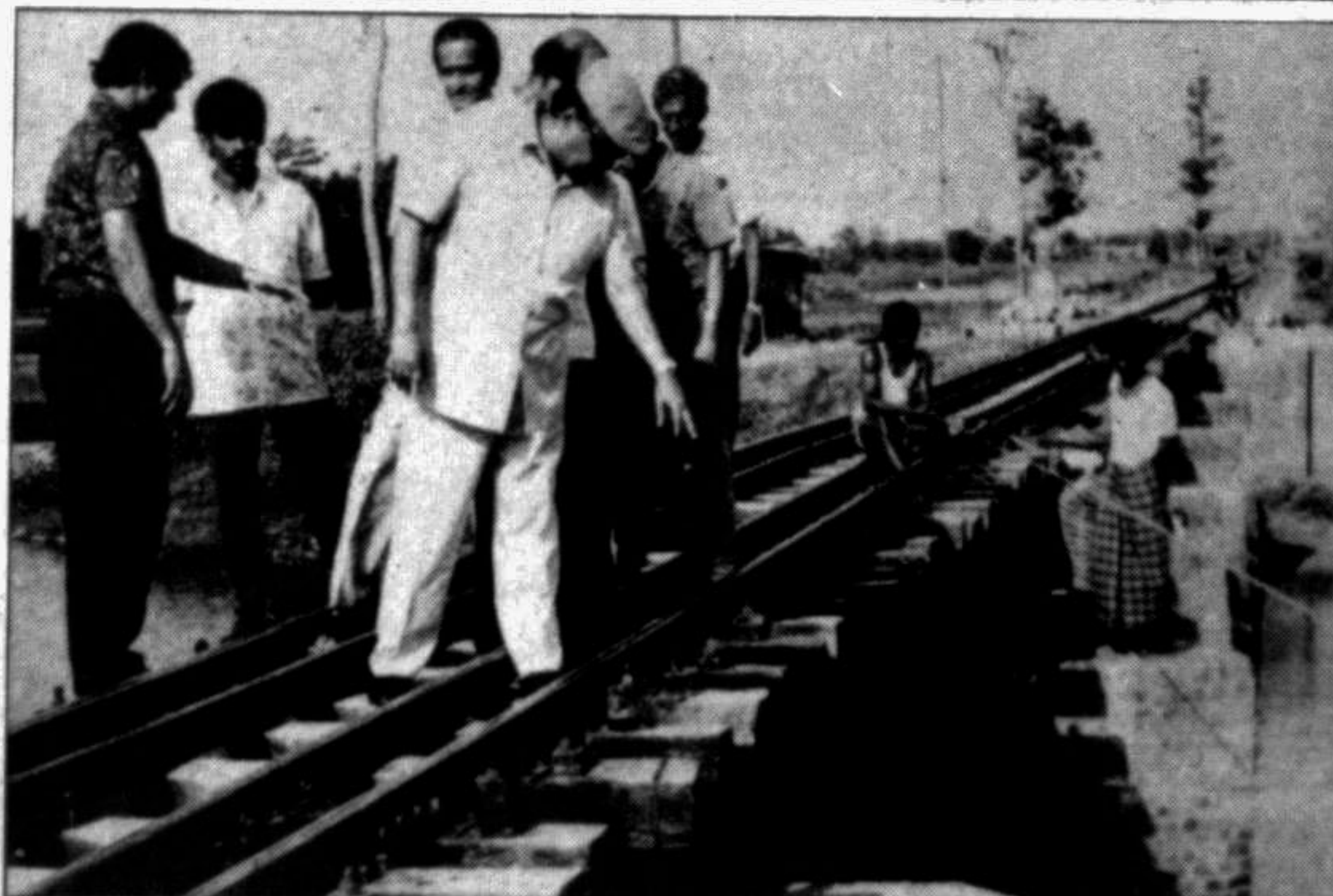
Railway Secretary Nurul Momen Khan inspecting the repair work of a rail bridge between Bharatkhal and Bonarpara Railway stations which went down following heavy downpour recently.
