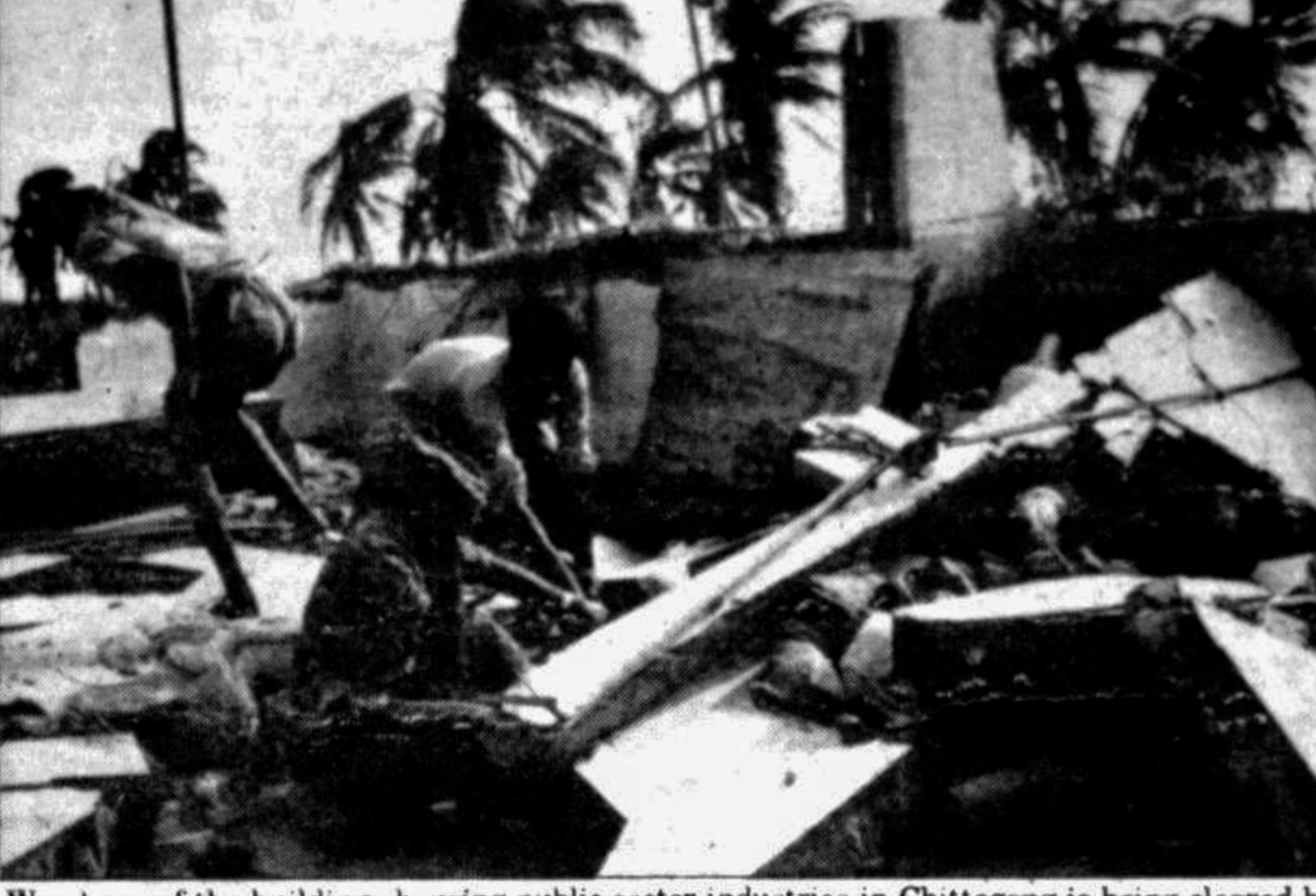
Wreckage of the buildings housing public sector industries in Chittagong is being cleared by rescue workers. The buildings collapsed following devastating cyclone of April 29. —Star photo
