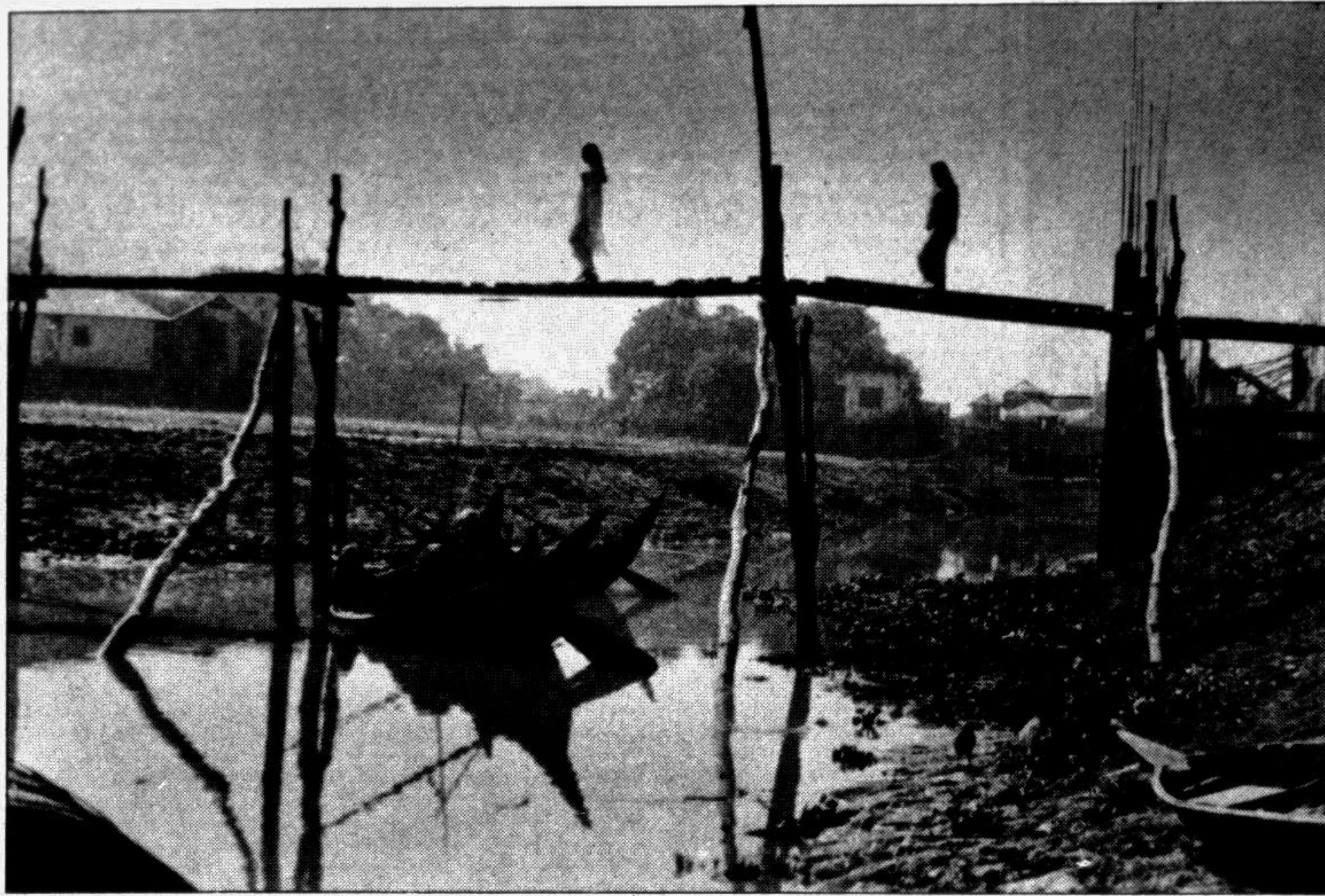
Construction of a concrete bridge started long ago over this canal at Keraniganj. But work remains suspended for fund shortage. People are thus compelled to undertake such hazardous crossing over this age-old broken wooden bridge.
