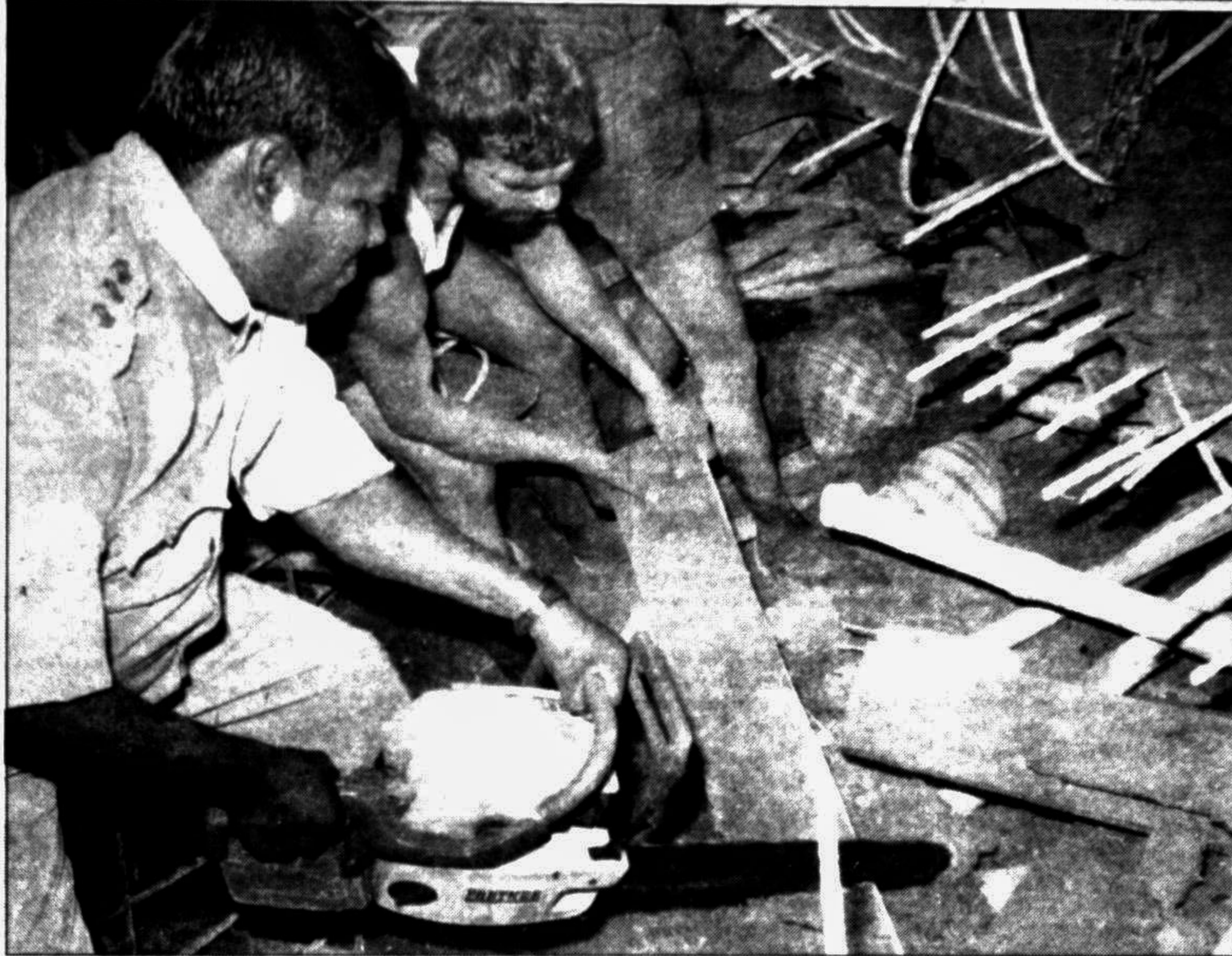
Workmen extricating a body through sawing steel plates at Sripur Textile Mills in Gazipur district on Wednesday. The roof of the mills collapsed following a norwester killing several workers. — Star photo
