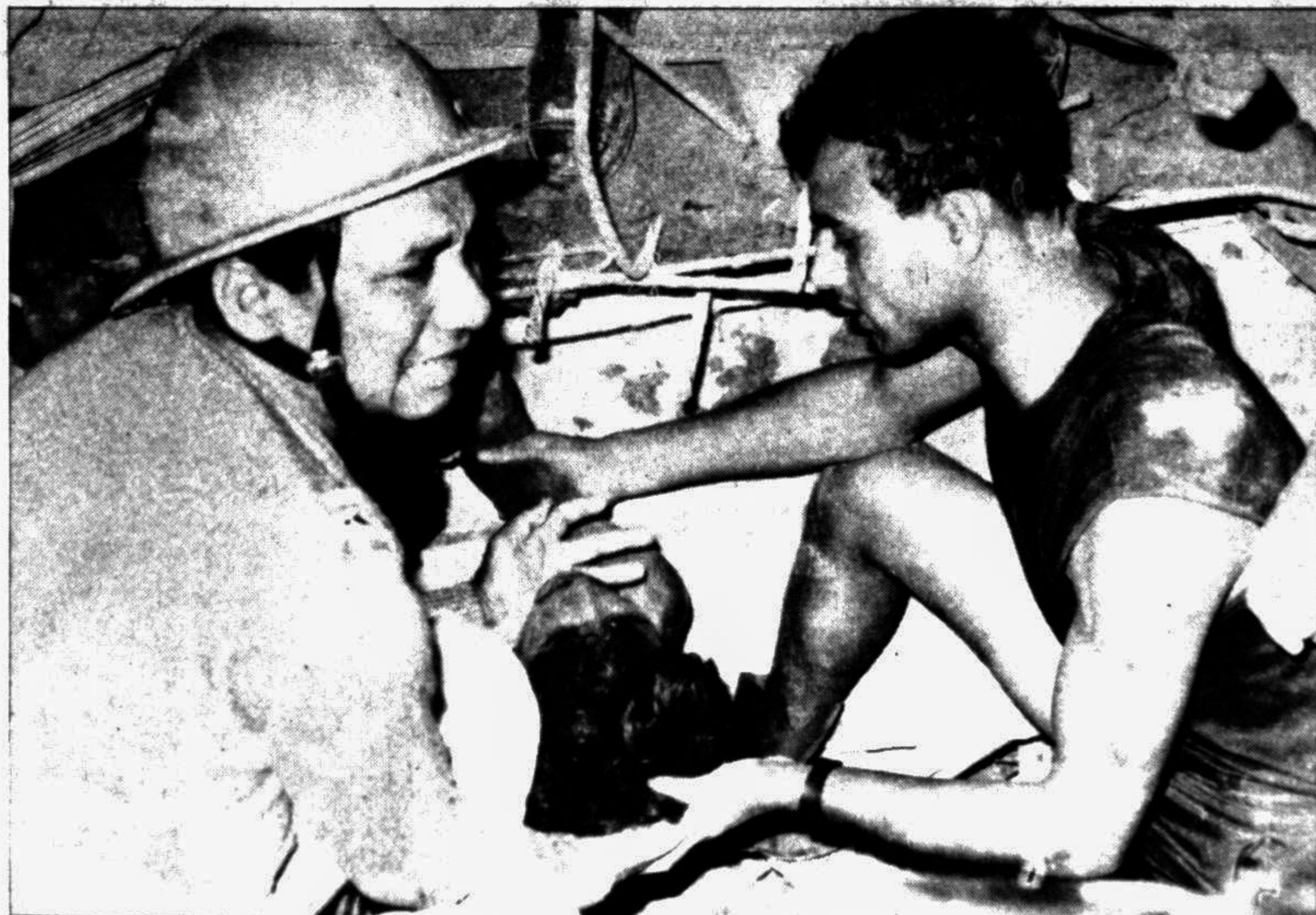
Body of a victim of Wednesday's nor'wester being rescued from the debris of an under-construction building of a textile mills at Gilarchala in Sreepur upazila of Gazipur district. — Star photo
