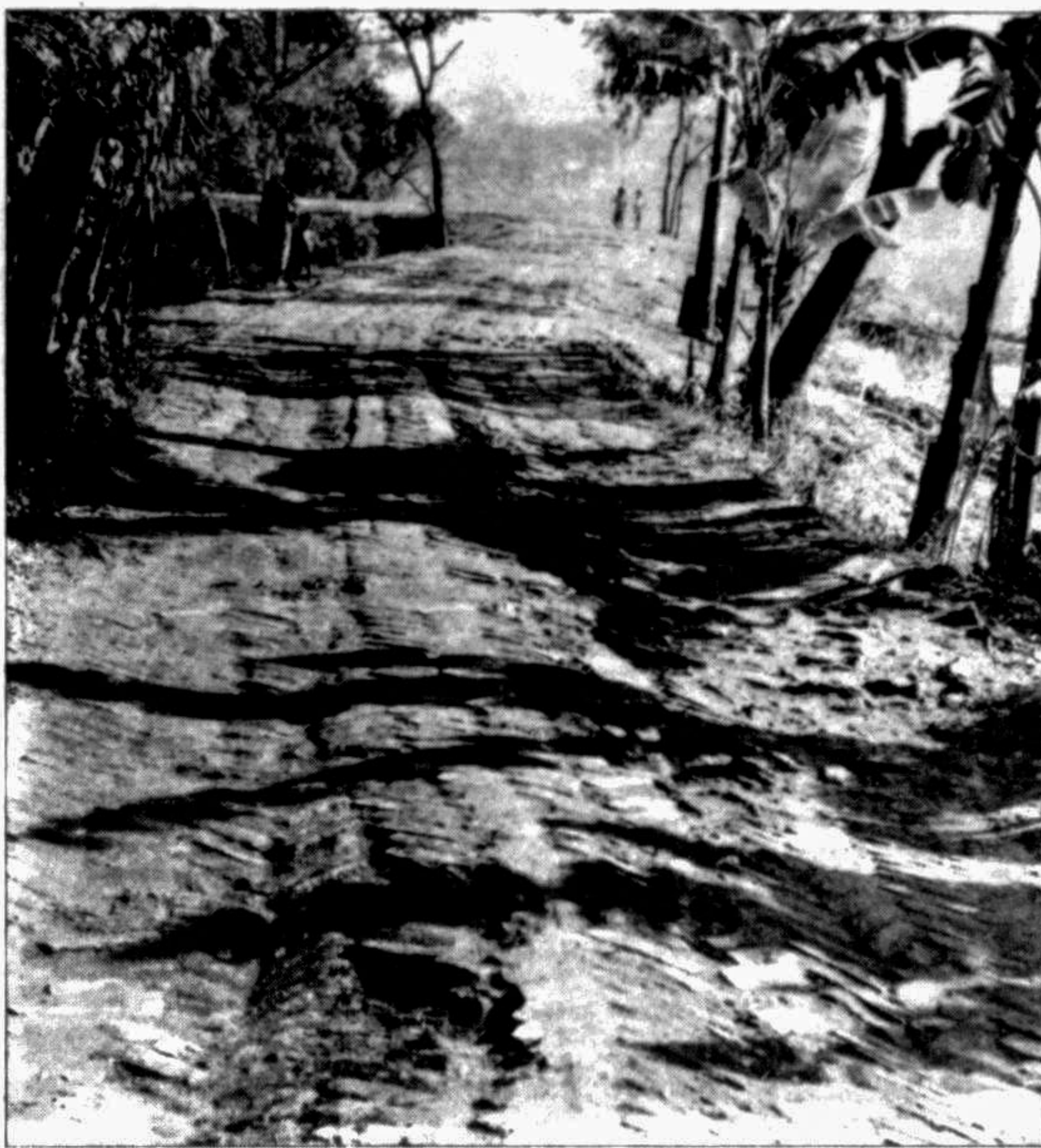
A dilapidated road at Lohajang upazila of Munshiganj district. — Star photo.
