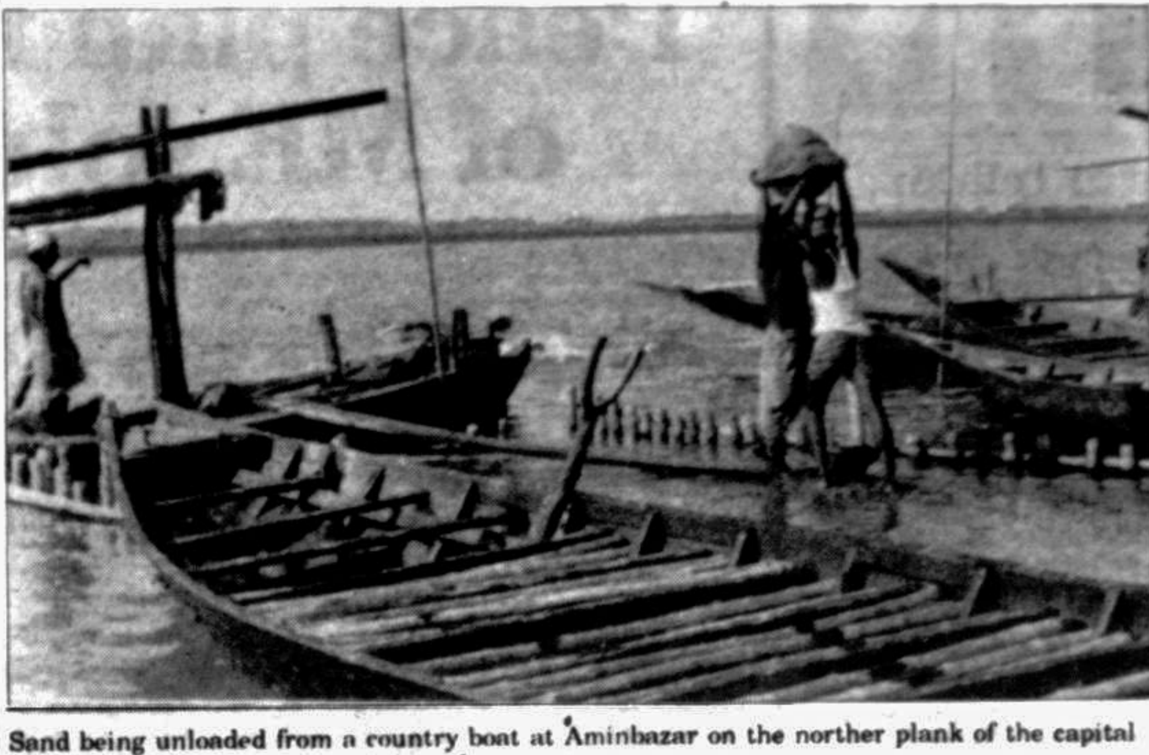
Sand being unloaded from a country boat at Aminbazar on the northern bank of the capital for earthfilling and construction works.
