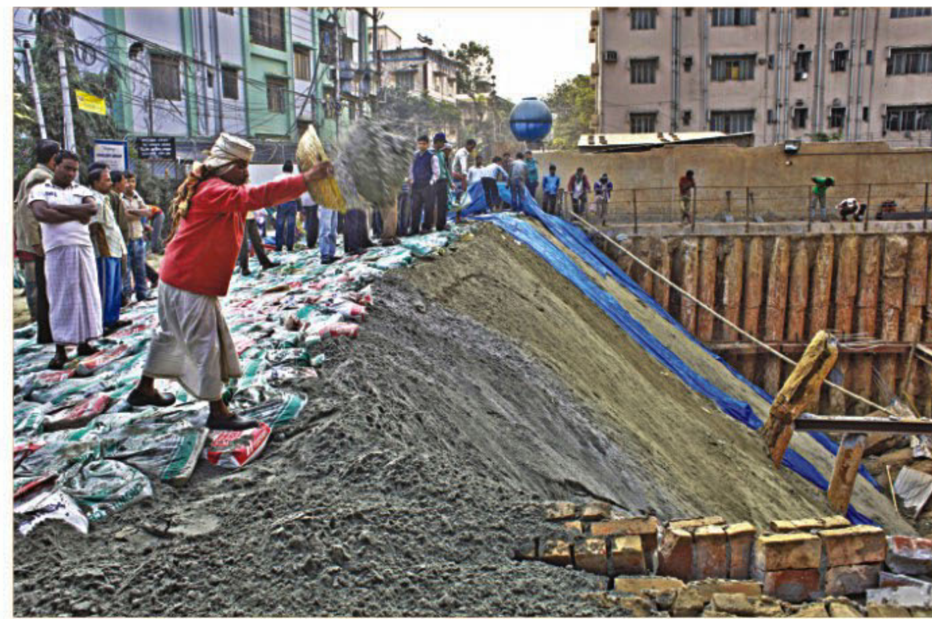
(Left) Sand being dumped at the portion where the Circuit House road collapsed on Monday. (Right) The construction site lacking adequate safety precautions puts the adjoining structures at the risk of collapse in the city's Purana Paltan. The photos were taken yesterday.
