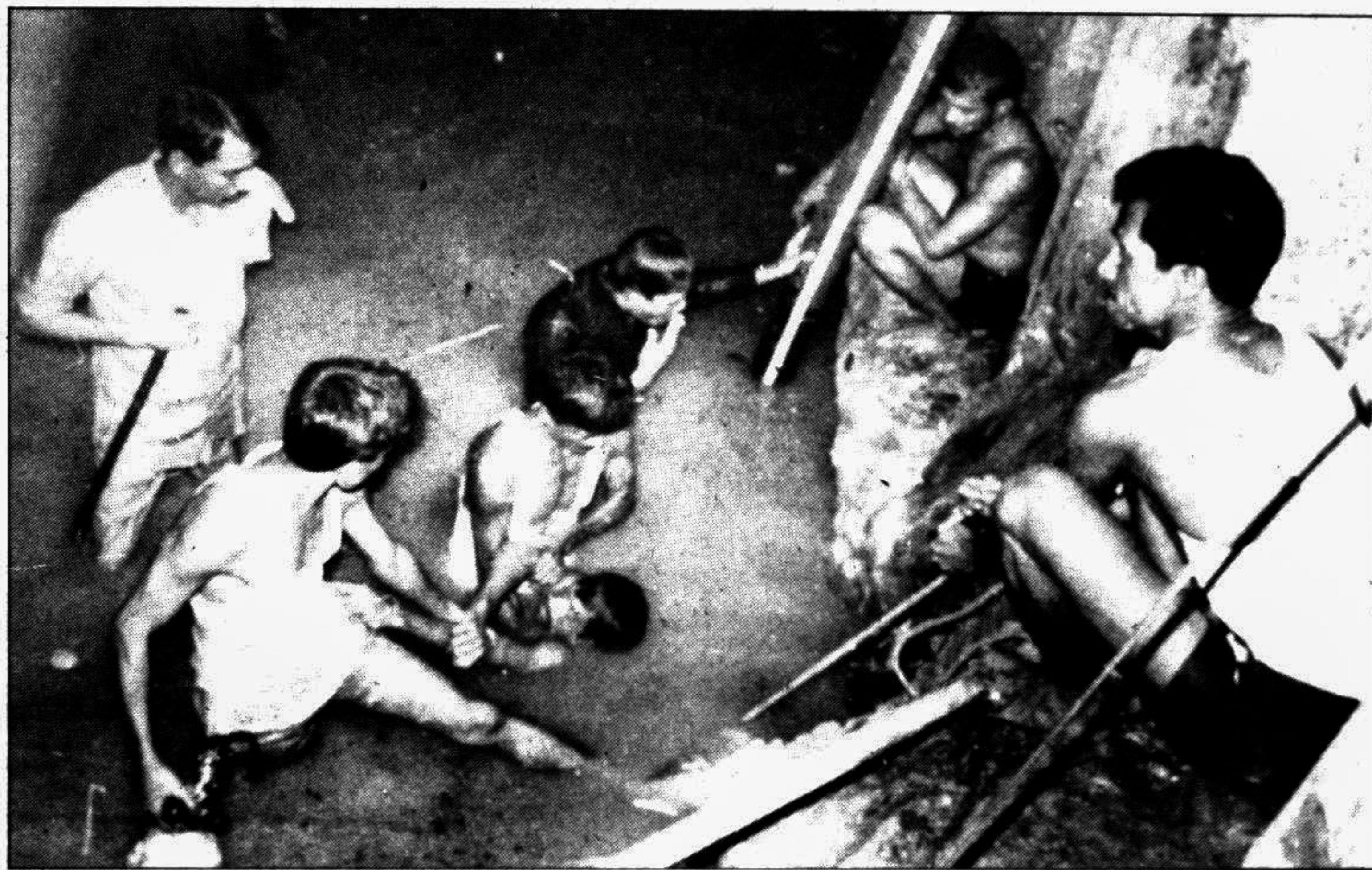
Fire Service personnel rescuing workers trapped when an underground sewerage pipe near Panthapath-Green Road intersection collapsed on Wednesday. —Star photo
