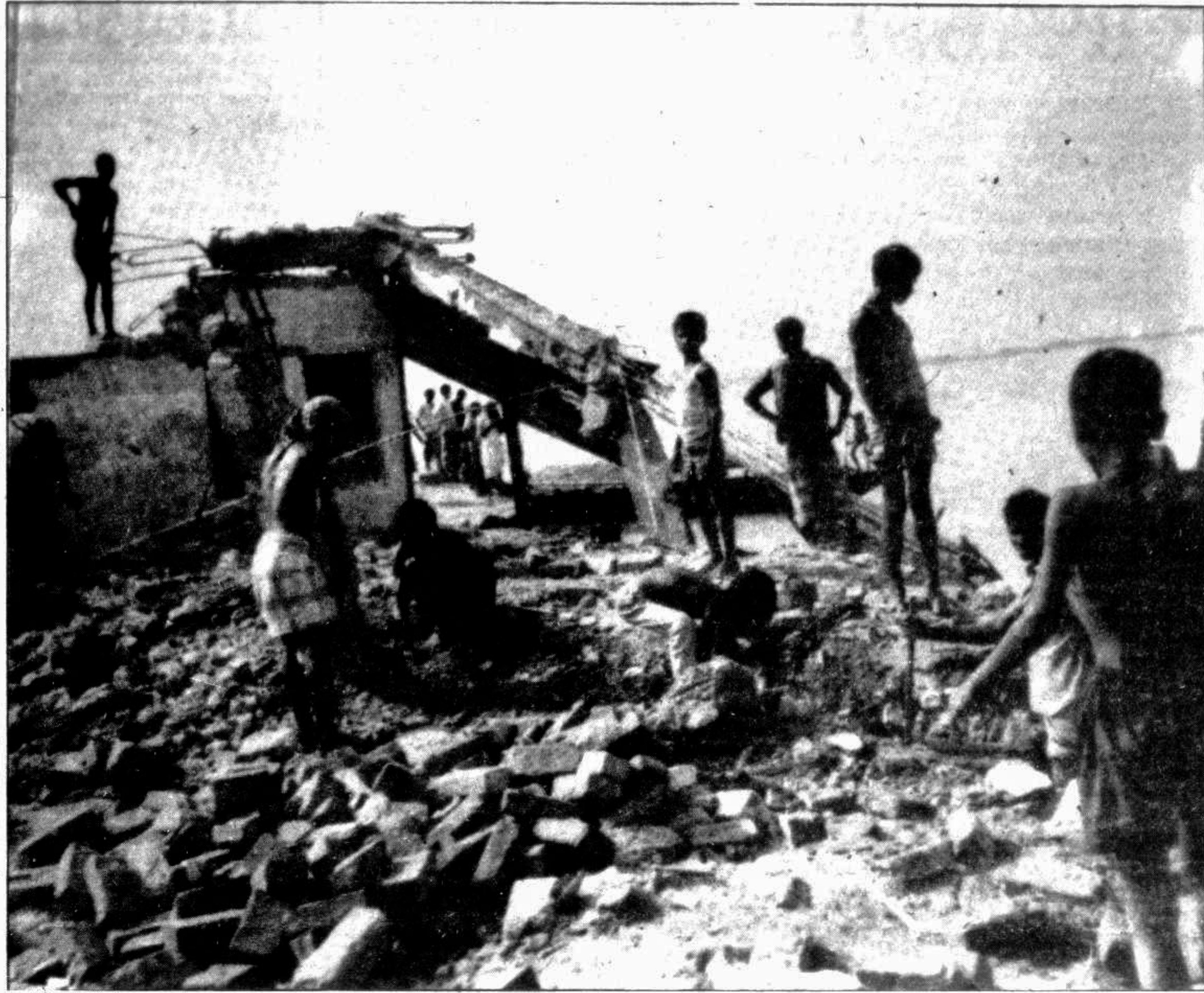
GAIBANDHA : The river Brahmaputra grabbed a vast tract of land at Fulchhari upazila. Photo shows a building dismantled to save the bricks and rods from the mighty river. —Star photo
