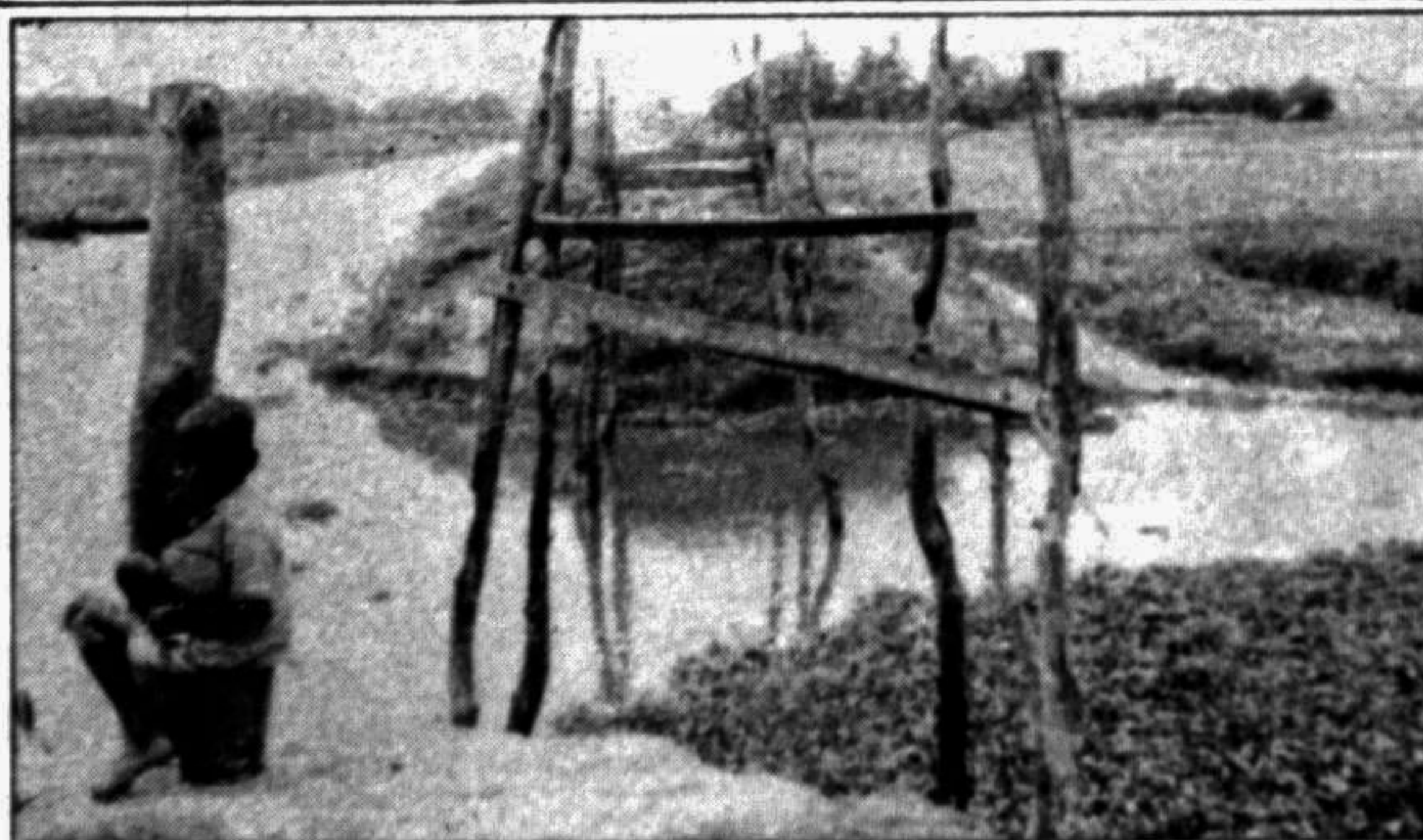
MUNSHIGANJ: This wooden bridge on Goltali Nowpara Hat Road damaged long ago is yet to be repaired.
