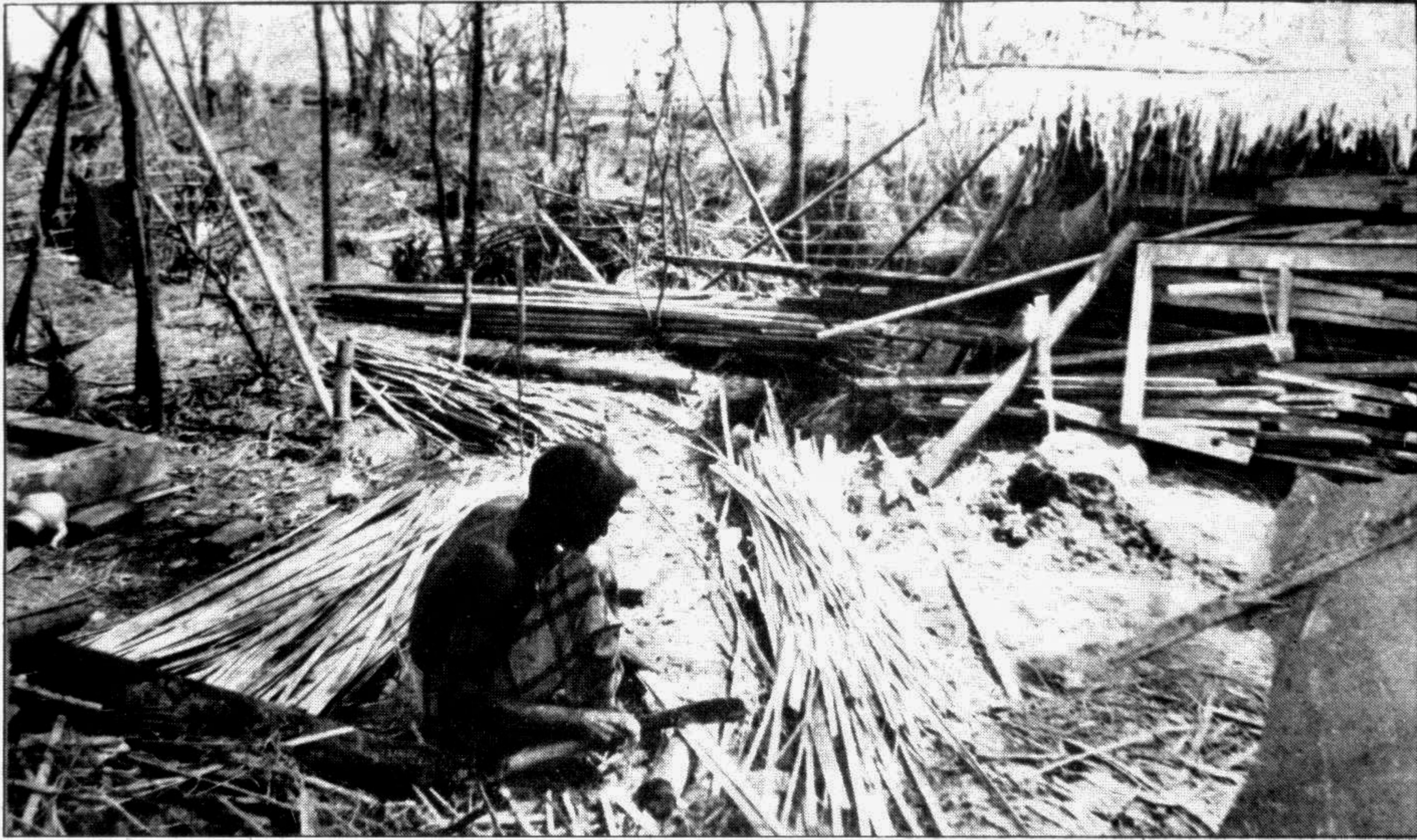
A survivor busy rebuilding cyclone-ravaged house at a village in Kutubdia. — Star photo
