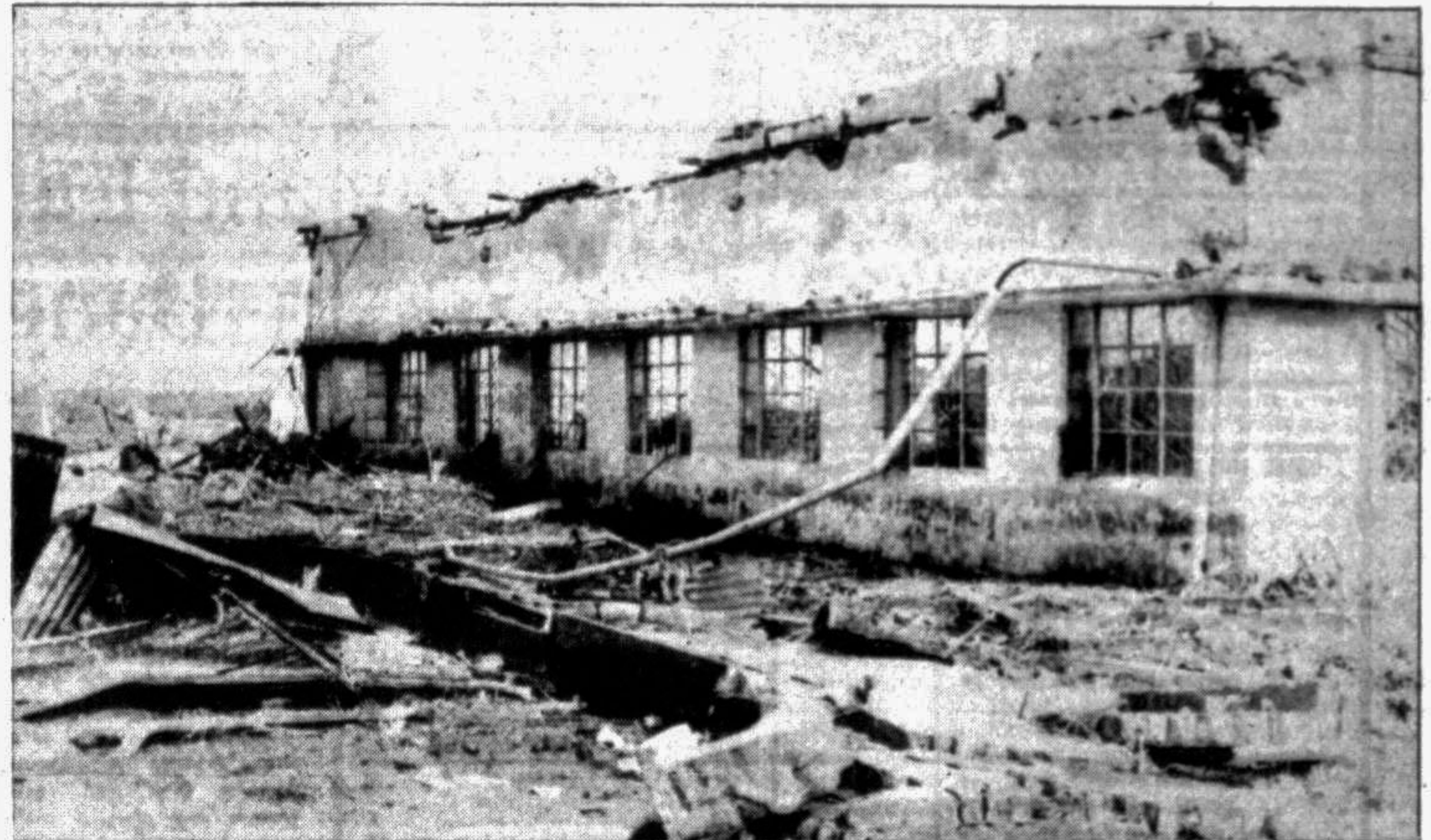
A strong concrete building at Kutubdia was no match for a cyclone having velocity of 250 kilometres per hour. Nobody still knows where hundreds, who took shelter in it, have gone. May be, they were flown off to the deep sea.
