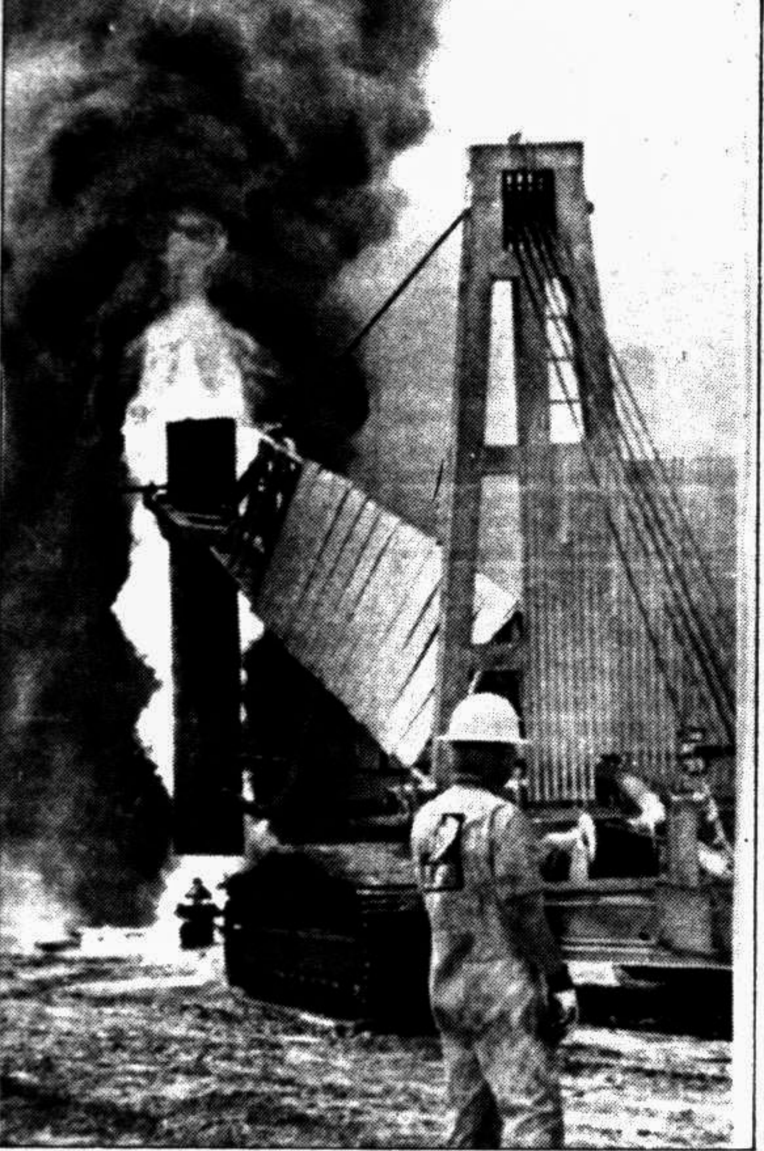
KUWAIT CITY: Men working for the US company "Boots and Coots" succeeded for the first time in extinguishing the flames from one of the many oil wells set ablaze by the Iraqis, by injecting air and nitrogen into a pipe held over the flame with the help of a crane in the Ahmadi oilfield some 20 km away from Kuwait City April 7. — AFP/UNB photo
