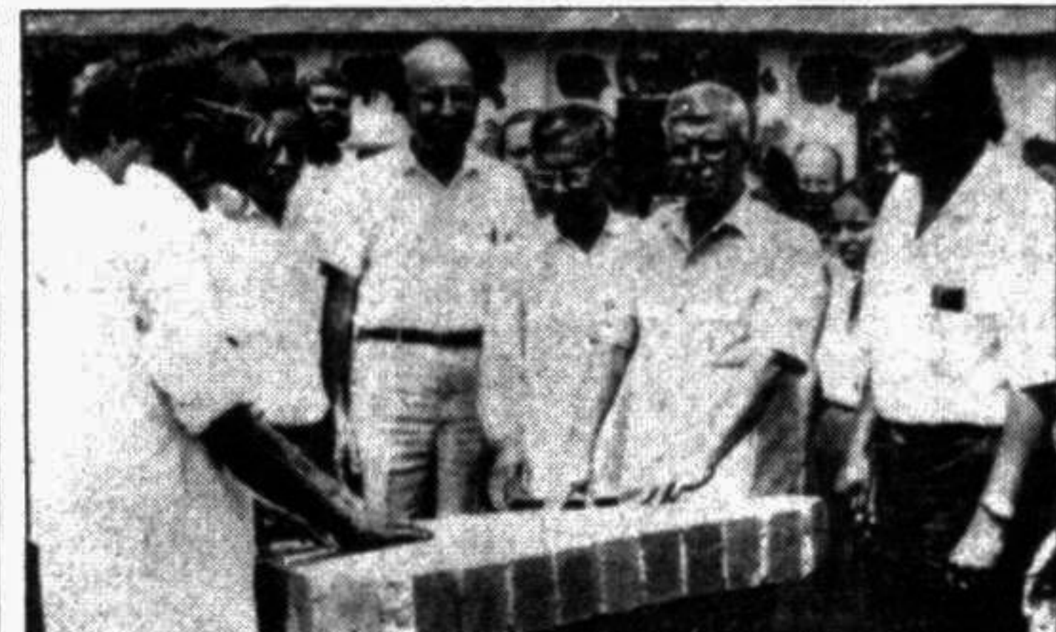
Prof. Dr. M. H. Khan, Vice-Chancellor, Bangladesh University of Engineering and Technology (BUET), laying foundation stone of a four storied building of Plassey Girl's High School administered by BUET, on Wednesday at Plassey.
