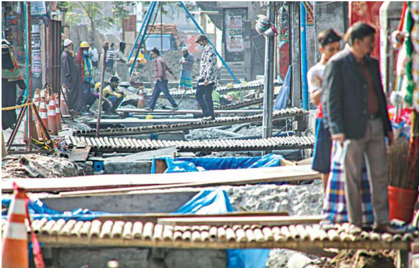
Dhaka South City Corporation has dug up a trench in Lalbagh Bazar Road for a development project causing immense sufferings to locals. They risk falling into the trench as they cross it with bamboo-made bridges that have no guard rails.
