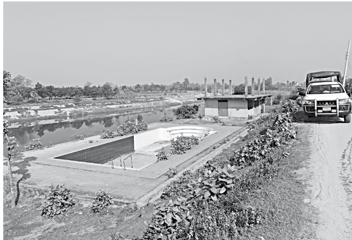
A mobile court yesterday demolishes this swimming pool, erected illegally occupying a portion of the Punarbhaba riverbank. A local influential man built this structure in Khalpara area of Dinajpur Sadar upazila about two and a half years ago.
