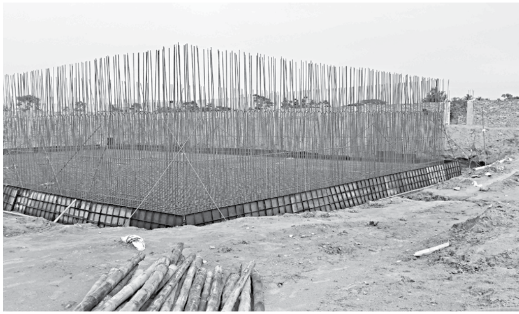
The under construction water treatment plant at Digraj intersection on Khulna-Mongla highway.
