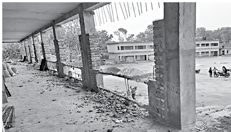
Local people vandalize this under-construction four storey schoolhouse of Dhanyakhola Secondary School under Benapole Port Police Station in Jashore on Sunday, bringing allegation of irregularities by the contractor concerned in the construction work.
