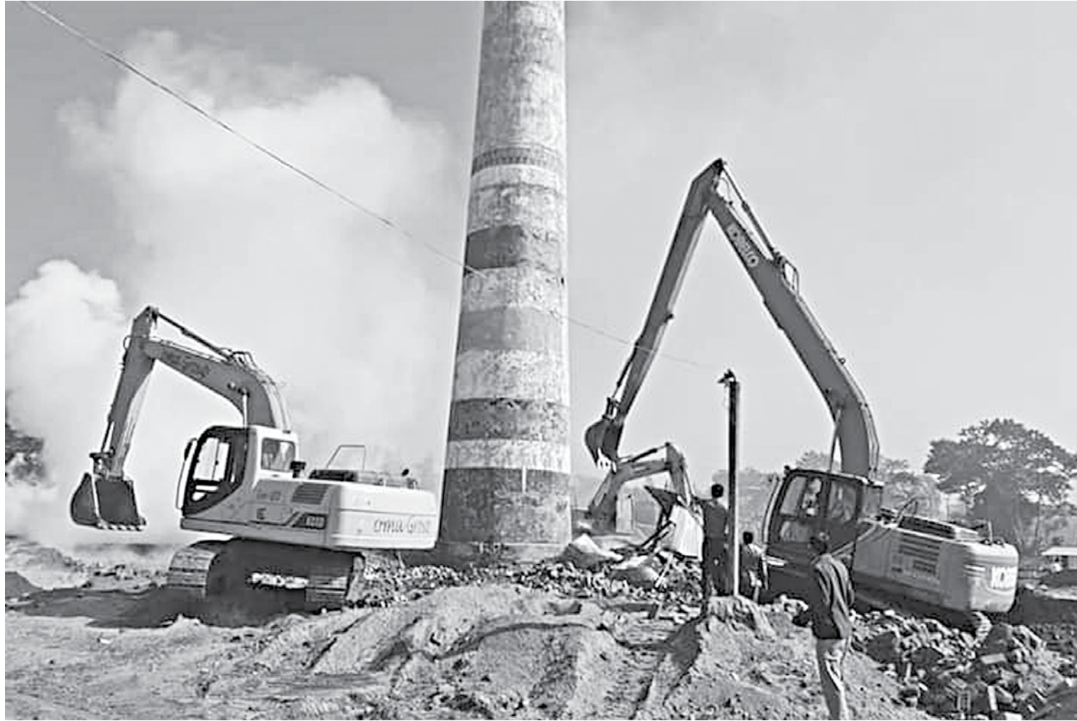
The High Court has ordered the Department of Environment in Chattogram to start a campaign to demolish all illegal brick kilns in the region. As part of a drive, DoE yesterday demolished three such kilns in Lohagara upazila.
