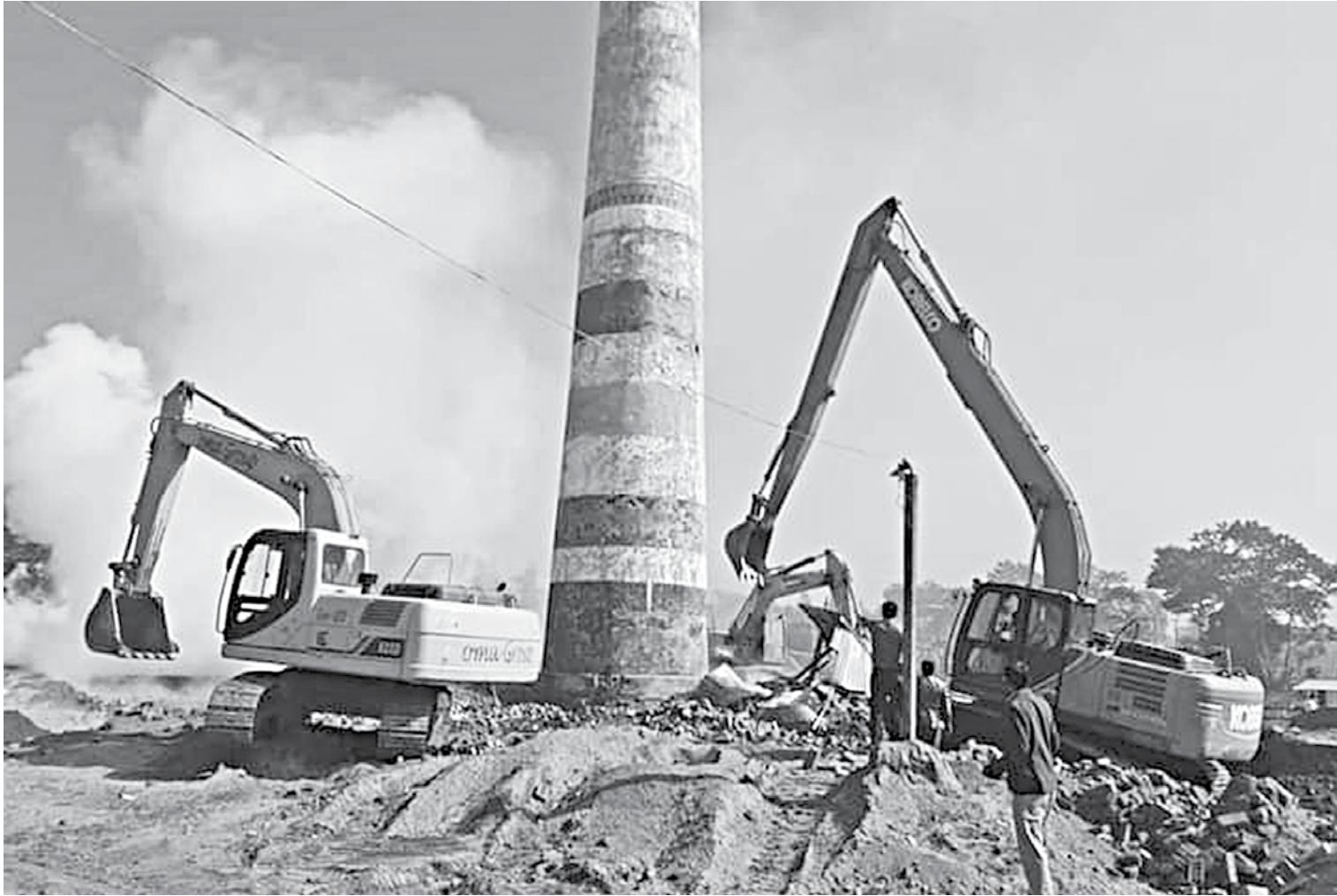
The High Court has ordered the Department of Environment in Chattogram to start a campaign to demolish all illegal brick kilns in the region. As part of a drive, DoE yesterday demolished three such kilns in Lohagara upazila. PHOTO: COLLECTED
