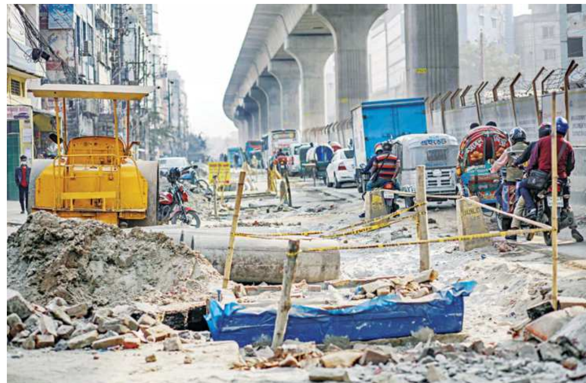
Traffic has been single file on Rokeya Sarani in the capital's Mirpur for the last three months since Dhaka Wasa excavated for development work a part of the road already narrowed down by work on the metro rail project. Vehicles could ply this road three abreast once. PHOTO: RASHED SHUMON
