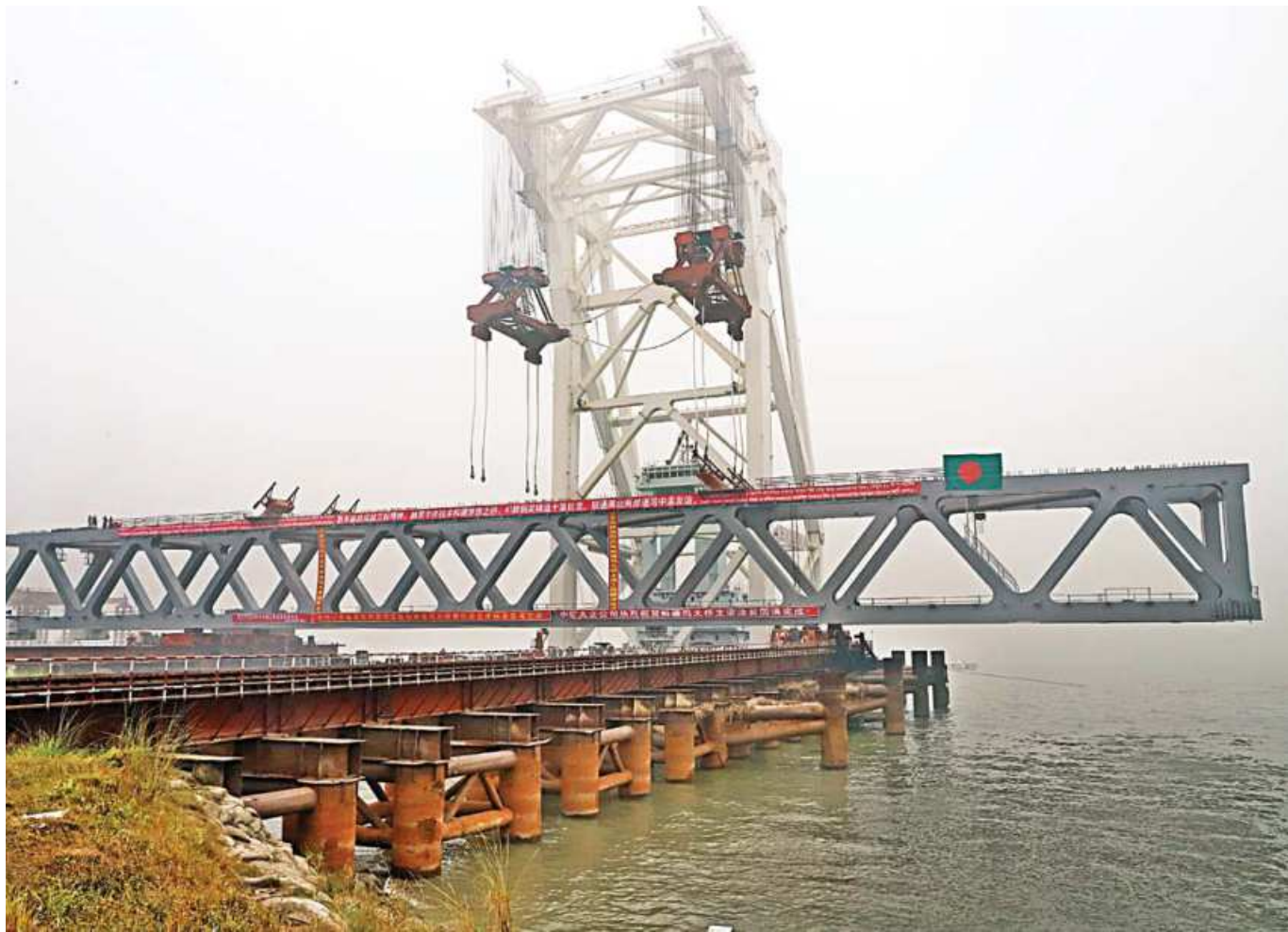
The last span of the Padma bridge is likely to be placed on the piers today, marking a milestone for the construction of the country's longest bridge. The photo was taken on Tuesday.
