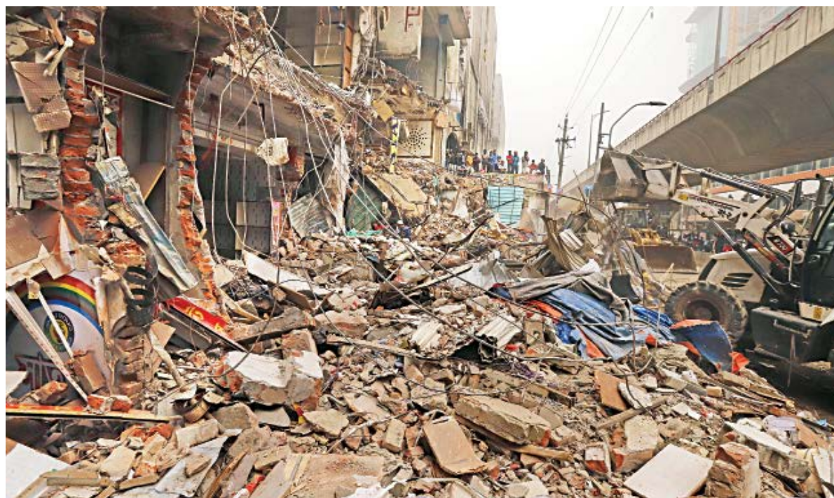
Rubble and debris of concrete by the road at Phulbaria after Dhaka South City Corporation authorities demolished illegal structures in the area yesterday.
