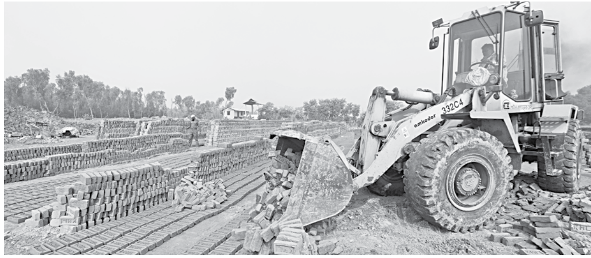
The illegal brick kilns ran for a decade as their owner managed to produce court stay orders. PHOTO: COLLECTED
