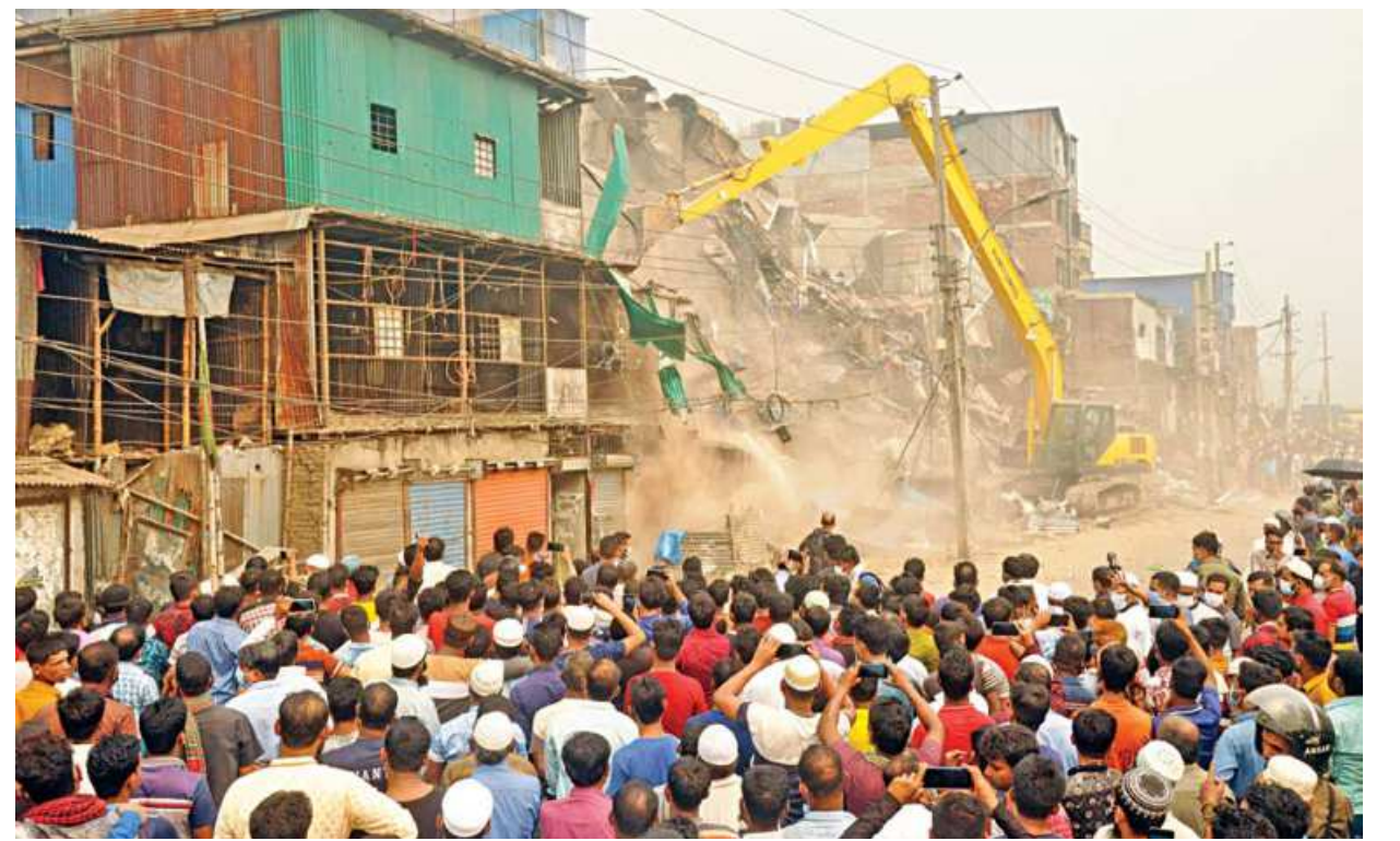
Many illegal tin-shed structures were demolished in yesterday's drive by Bangladesh Inland Water Transport Authority at Old Dhaka's Islambagh and Kamalbagh areas near Buriganga River. Shopkeepers and residents had taken their belongings out before the eviction took place.
