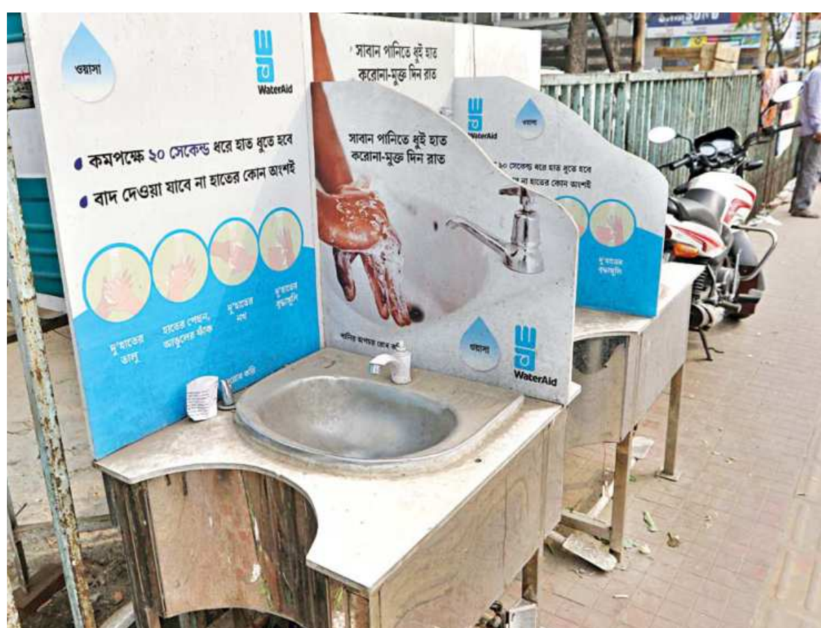
Sinks installed for washing hands at the capital's Karwan Bazar on Kazi Nazrul Islam Avenue appear to have been not used for quite a while. There was no water supply or soap there when this photo was taken yesterday. Coronavirus infections and deaths caused by the pathogen are on the rise.
